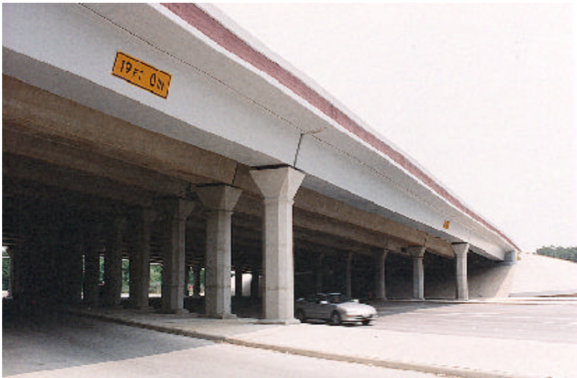
Scanning studies accelerated the use of high-performance concrete to build longer-lasting bridges that suffer less damage from traffic and weather.
