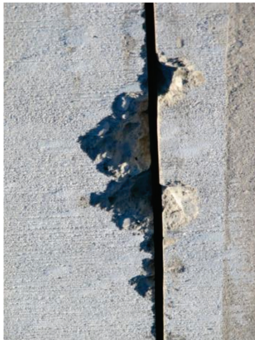
Figure 9 – Excessive Joint Raveling
