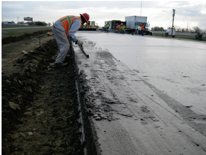
Figure 10 – Non-uniform Concrete Leads to Paving Issues
