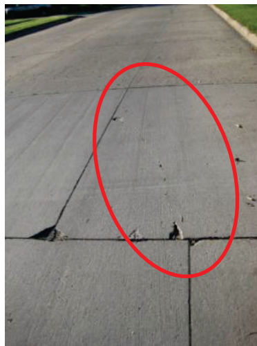
Figure 8 – Example of Poor Joint Detailing
