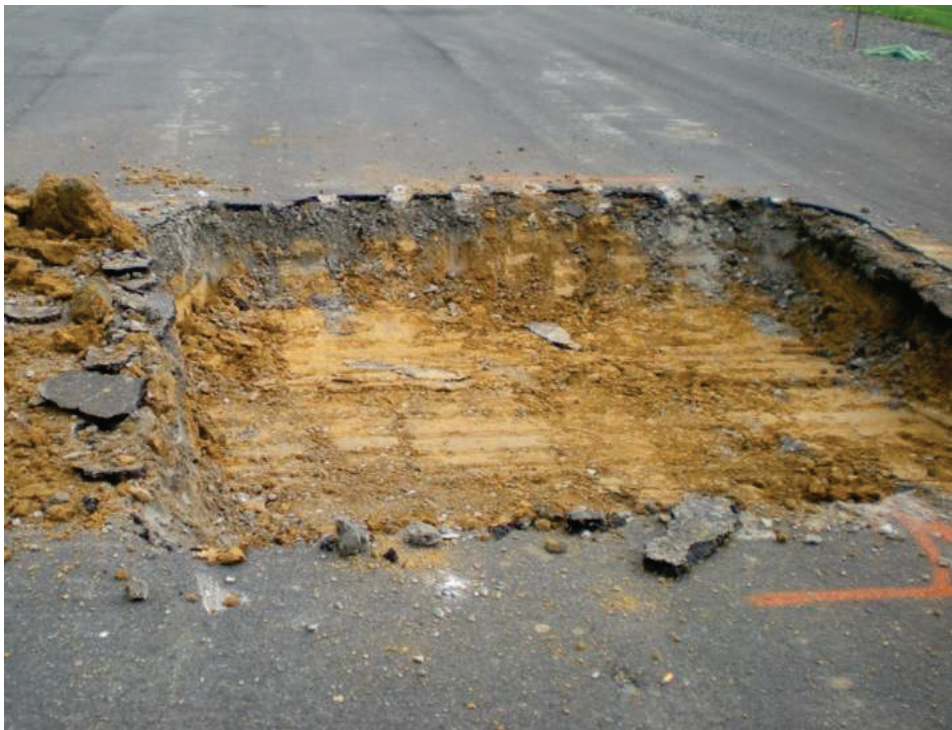
Figure 20 – Subgrade/Subbase Failures Must Be Repaired to Achieve Uniform Support
