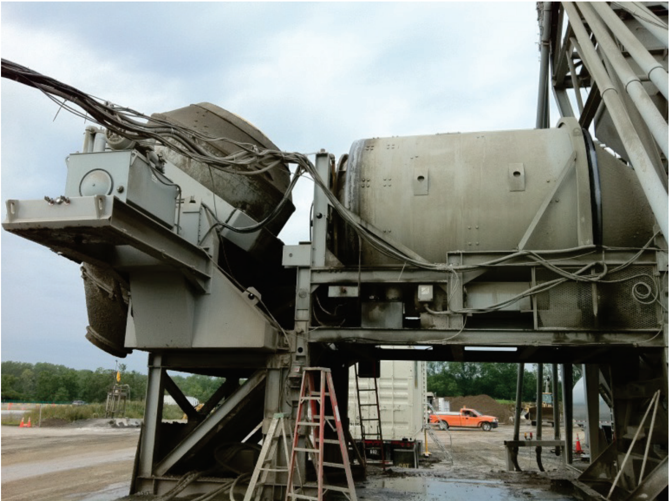
Figure 32 – Proper Plant Set-up and Maintenance is Critical to Providing Uniform Concrete
