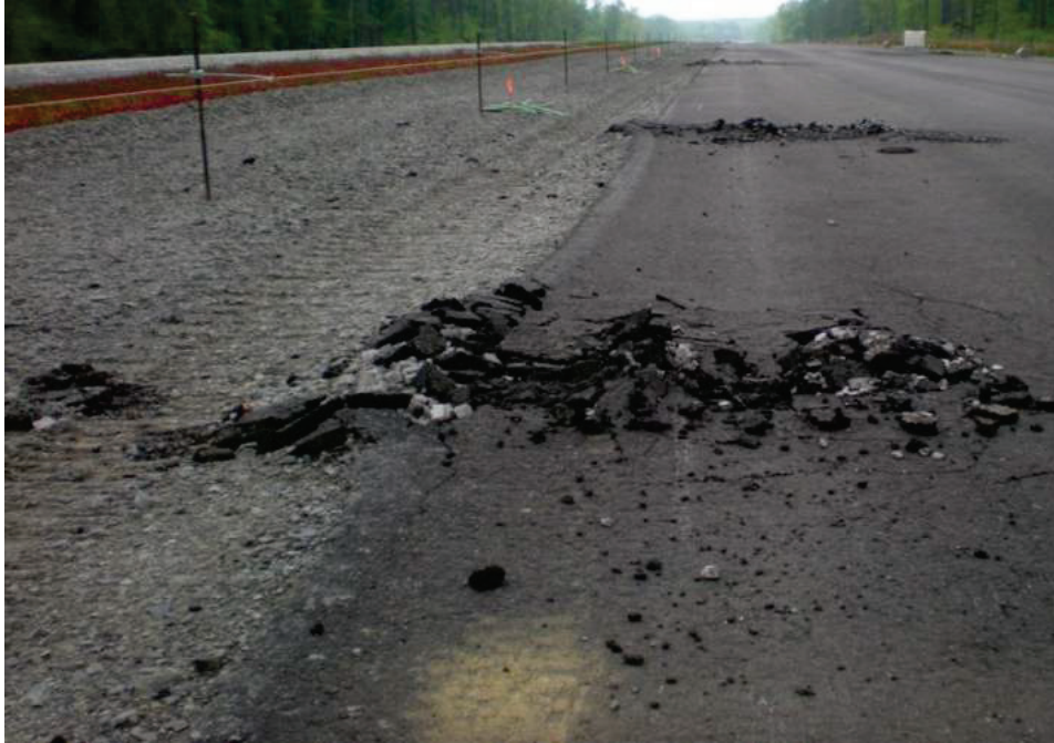
Figure 19 – Identify Subgrade/Subbase Failures
