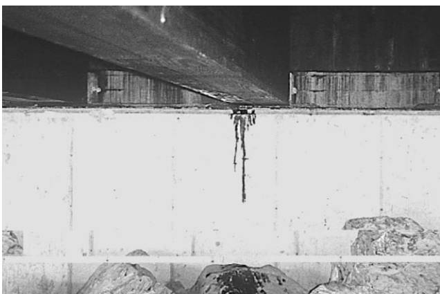
Figure 26 —Creosote staining of concrete abutments resulting from preservative leaching.
