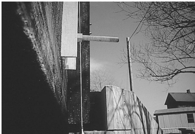
Figure 24 —“Toe in” of exterior beams resulting from tensioned diaphragms.
