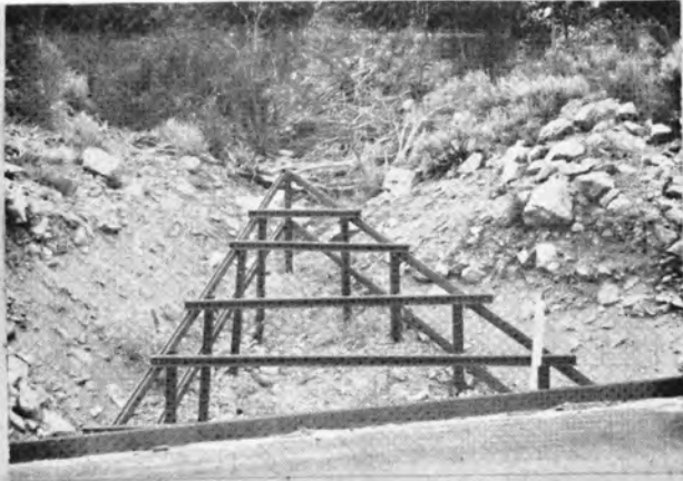
Figure 1. Steel rail debris deflector for large rock.
