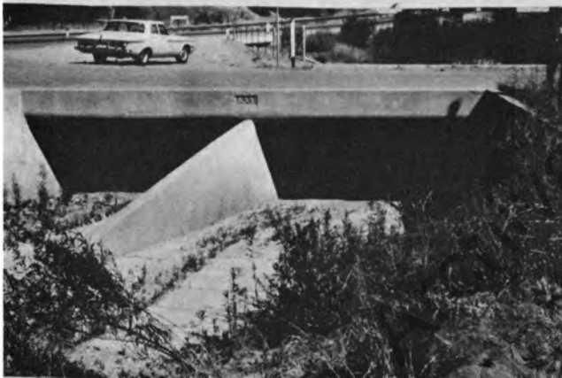
Figure 41. Concrete debris fin with sloping leading edge as extension of center wall.
