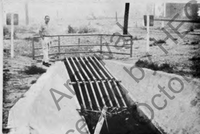
Figure 26. Pipe grill debris rack. Vertical fence at downstream end to prevent debris from spreading over ponding area.
