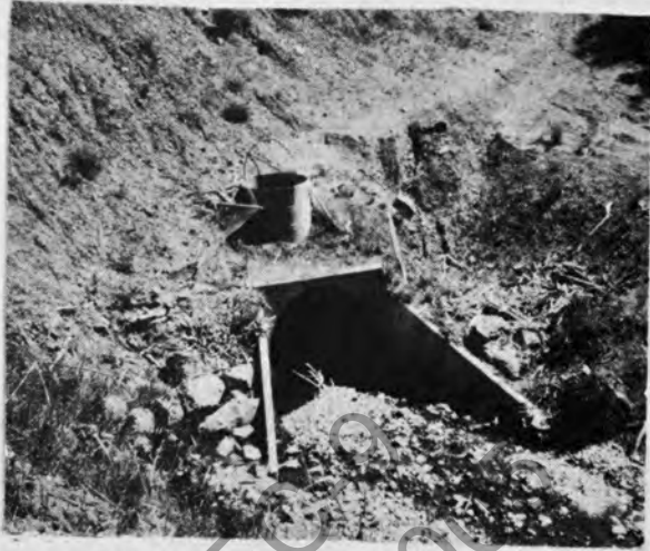
Figure 33. Metal pipe debris riser placed during initial construction of culvert provides relief in case the latter becomes plugged. (See Fig. 34.)
