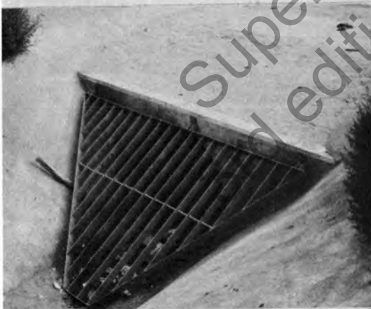
Figure 19. Hinged steel debris rack in urban area. Due to nature of debris and possible entry by children, bar spacing is close.
