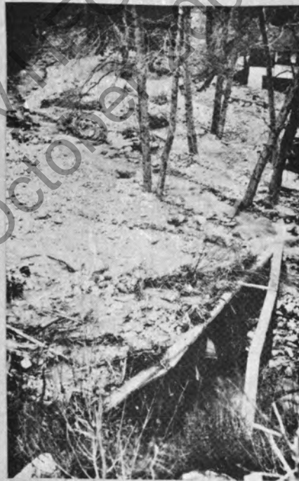
Figure 13. Timber pile debris deflector protected culvert during heavy floods. Nearby culverts without deflectors were plugged.
