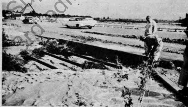
Figure 7. Installation shown in Figure 6 during flood; function well under heavy debris flow.
