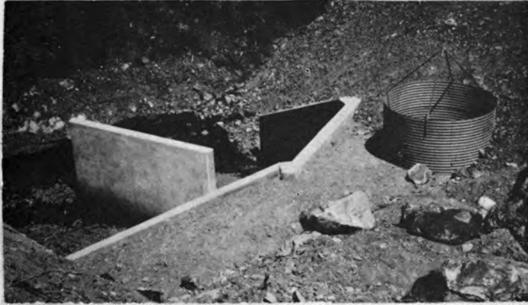
Figure 45. Debris fin and metal pipe debris riser in conjunction with single barrel culvert.
