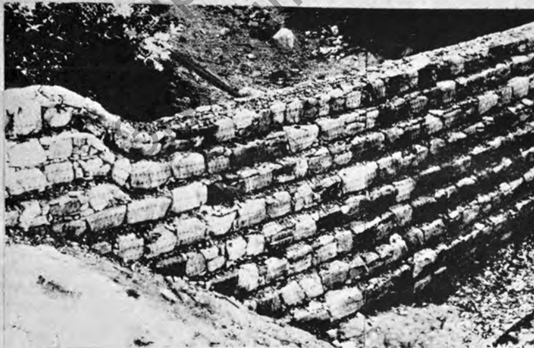
Figure 47. Debris dam of rock and wire.
