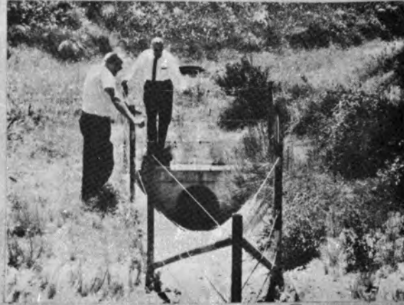
Figure 9. Wire and post debris deflector for light floating debris.
