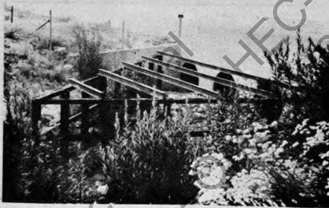
Figure 6. Steel rail debris deflector for battery of culverts (See Fig. 7).
