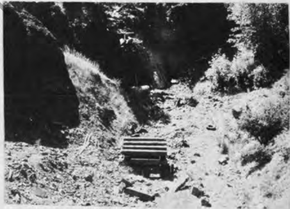
Figure 35. Timber debris crib in ideal location, i.e., high roadway embankment and large settling basin.
