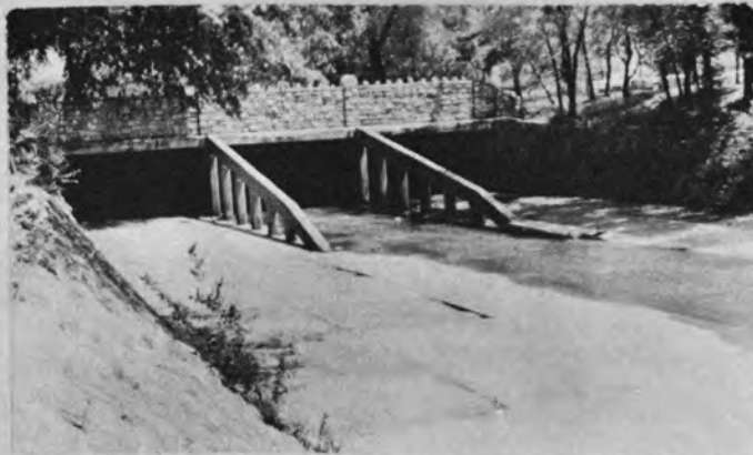
Figure 40. Concrete debris fins with sloping leading edges as extensions of culvert walls.
