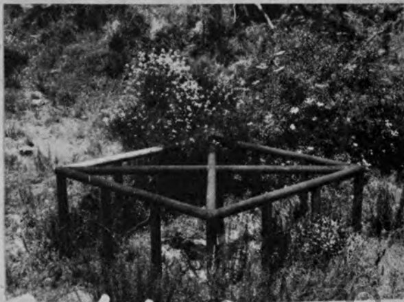
Figure 29. Post debris rack placed over entrance to metal pipe debris riser after latter had caused deposition.
