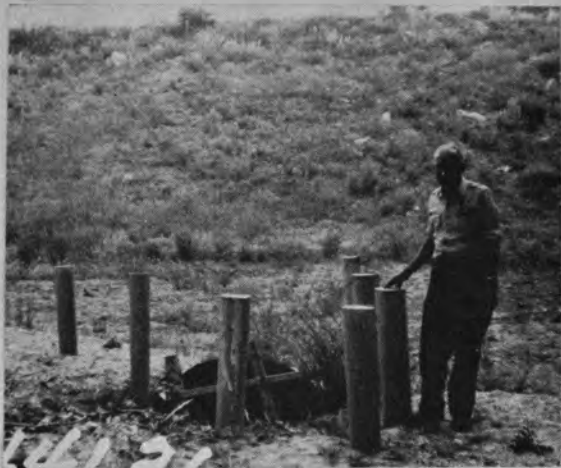
Figure 28. Metal pipe debris riser, with posts to deflect boulders, installed by maintenance forces on 45^\circ angle to vertical.
