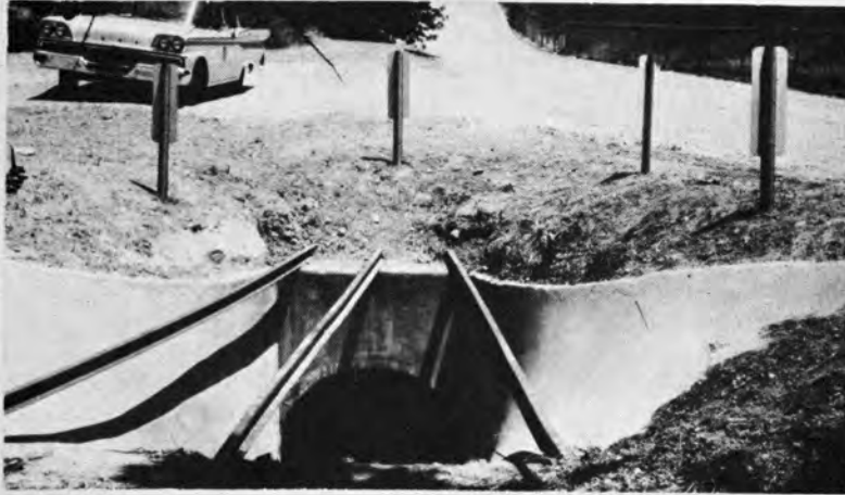
Figure 14. Rail debris rack over sloping inlet. Heavy debris and boulders ride over rack and leave flow to culvert unimpeded.
