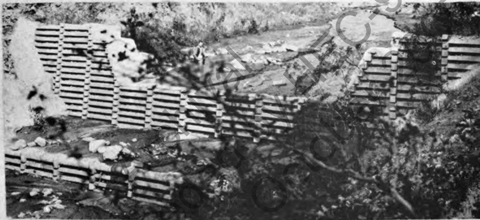
Figure 50. Debris dam of precast concrete sections fabricated to enable placement in interlocking fashion.
