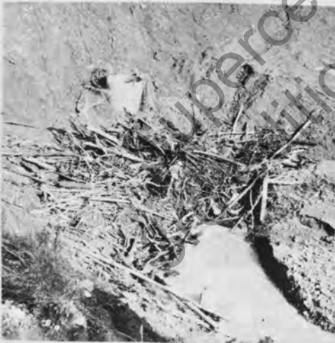
Figure 34. Installation shown in Fig. 33 after flood. Riser carried heavy flow during flood. Fence partially surrounding riser of no value for debris control. (Note man at center of photograph.)
