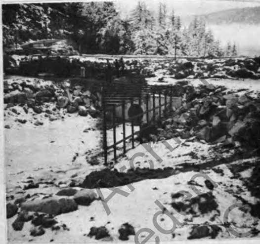
Figure 2. Steel rail debris deflector.
