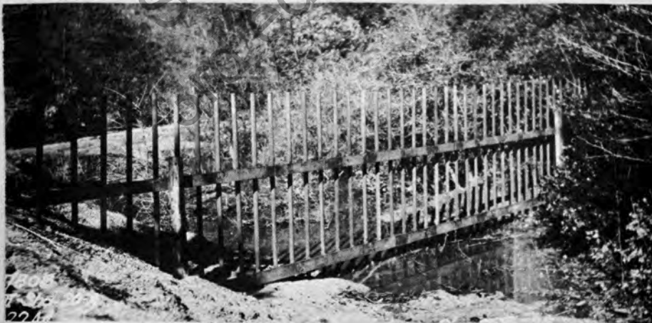
Figure 16. Post and rail debris rack, in place for 35 years, for light to medium floating debris installed 100' upstream of culvert.
