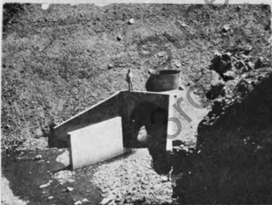
Figure 43. Concrete debris fin and metal pipe debris riser in conjunction with single corrugated metal pipe culvert.
