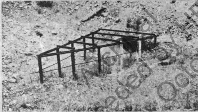
Figure 10. Steel rail and cable debris deflector. Cable's flexibility more desirable than rail's rigidity in boulder areas.
