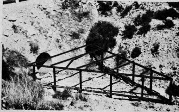
Figure 5. Steel rail debris deflector.
