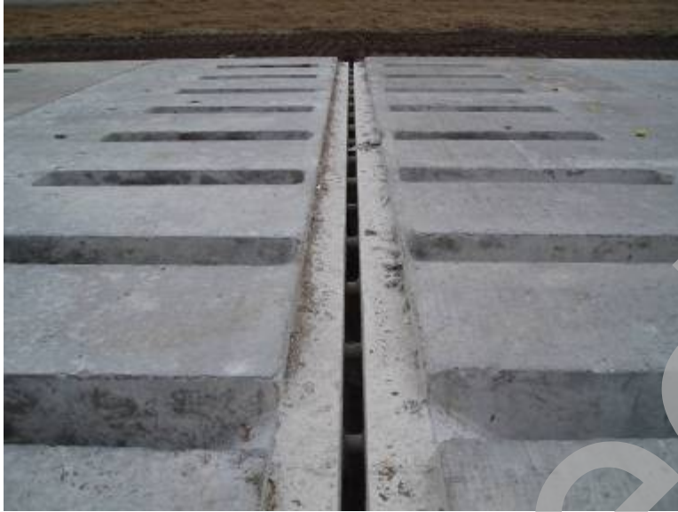
Figure 40. Photo. Expansion joint after being pulled open during the post-tensioning operation. (photo from MoDOT).
