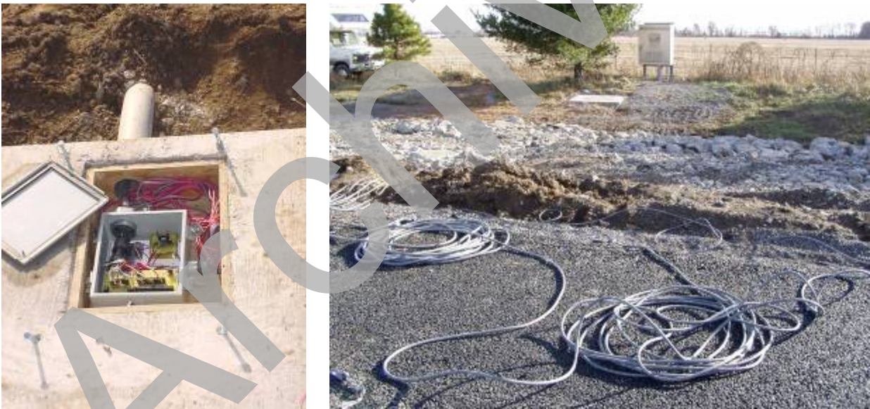
Figure 58. Photo. Junction box within an instrumented precast panel (left) and instrumentation cabinet next to the project site for collecting and uploading data (right).
