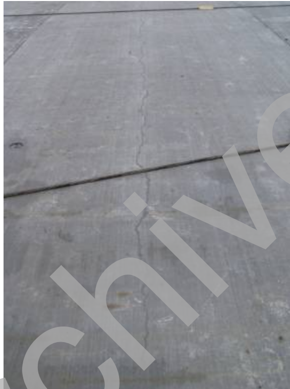
Figure 28. Photo. Typical hairline longitudinal crack observed at the fabrication plant (photo taken after precast panel was delivered to the project site).
