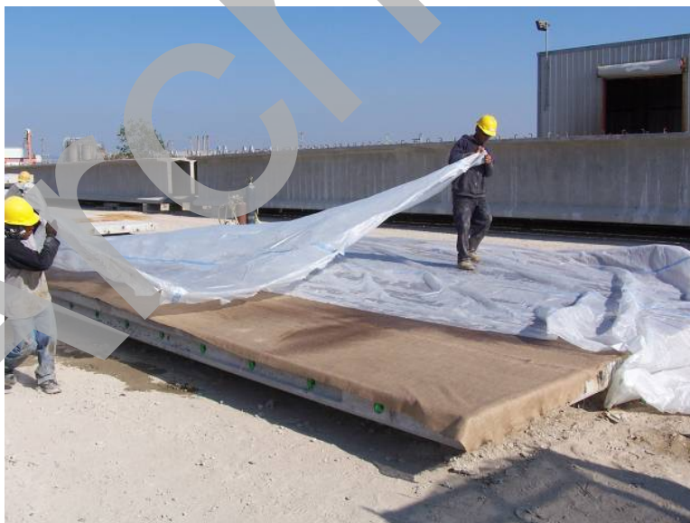
Figure 25. Photo. Wet burlap mat curing of the precast panels after removal from the forms.
