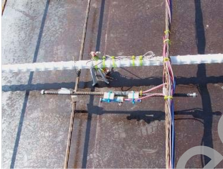
Figure 57. Photo. Instrumented rebar and vibrating wire strain gages for measuring concrete strain.
