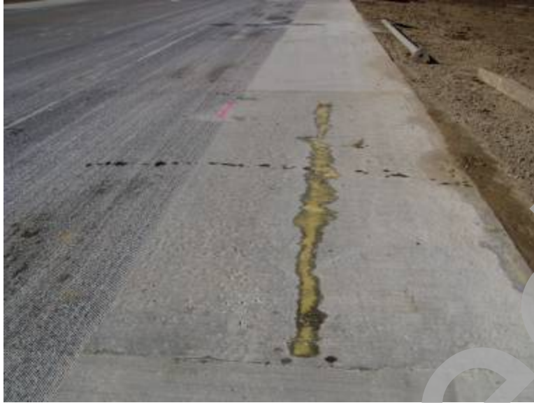
Figure 29. Hairline transverse crack in the shoulder after epoxy sealing (photo taken after panel was installed on site).
