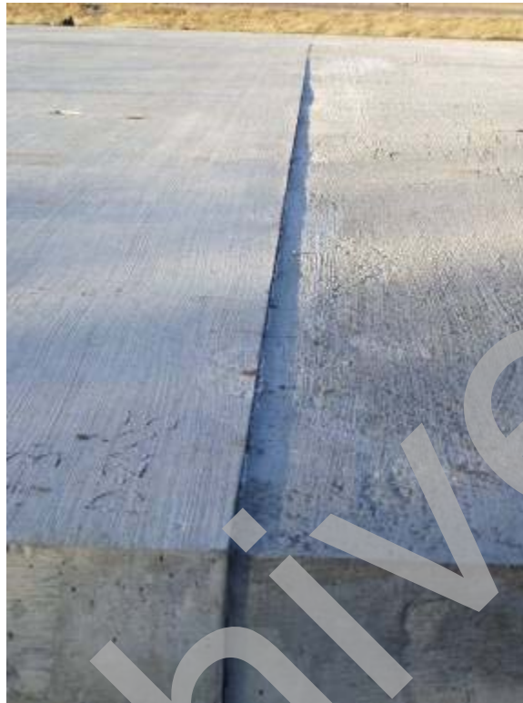
Figure 48. Photo. Faulted joint observed in the shoulder region.
