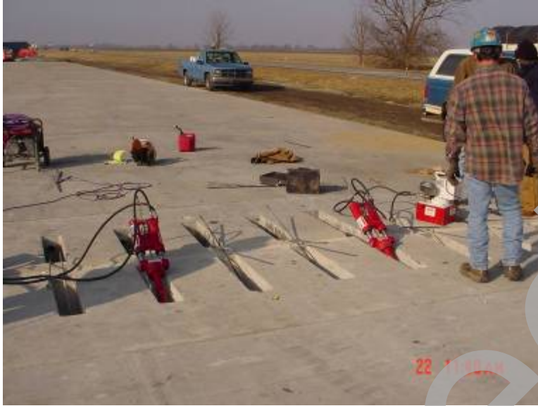
Figure 39. Photo. Final longitudinal post-tensioning completed using two post-tensioning rams (photo from MoDOT).
