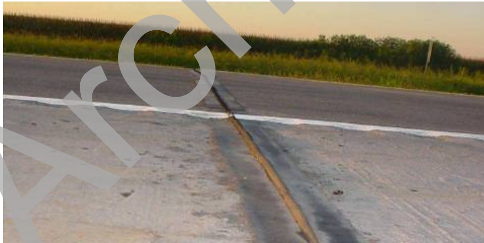
Figure 44. Photo. Joint sealant protruding from the surface of the pavement during under summer climatic conditions. (18)
