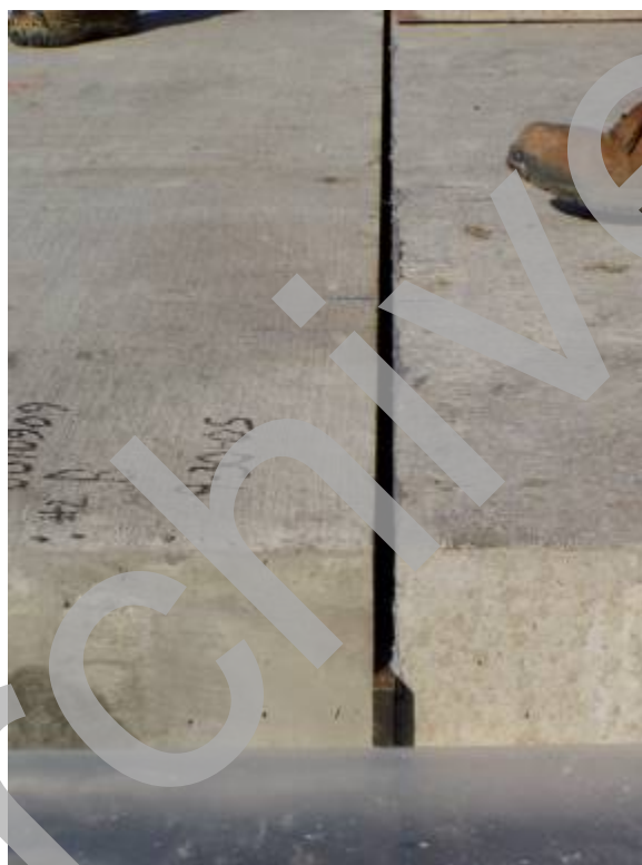
Figure 47. Photo. Shims at the outside edge of the pavement used to correct centerline alignment.
