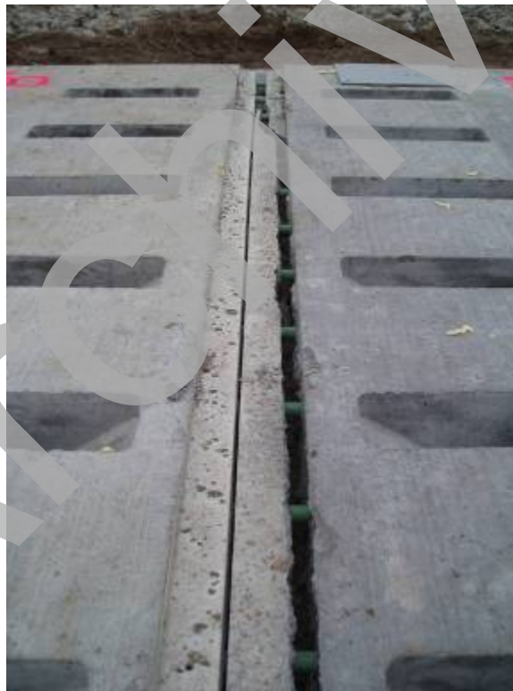
Figure 41. Photo. Expansion joint No. 4 after fracturing during the post-tensioning operation. (photo from MoDOT).
