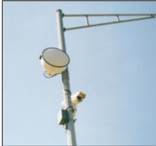
Freeway surveillance camera and antenna at intersection
