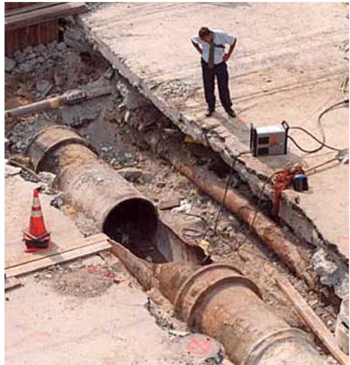
Figure 8. The Water Main Break
