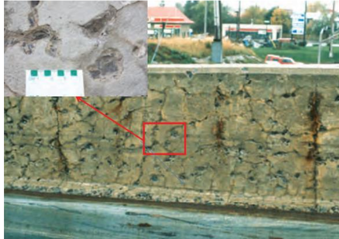
Figure 1.9: Map-cracking along with several pop-outs caused by particles of shaly limestone (from Thomas et al., 2013)
