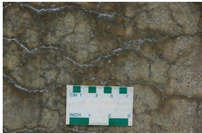
Figure 1.10: Surface discoloration and exudation associated with cracks (from Thomas et al., 2013).
