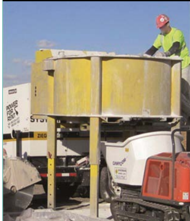
Figure 3. Portable concrete pan mixer preparing UHPC for placement during the construction of the field-cast connections.
