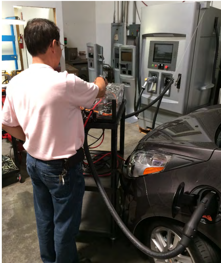
Figure 15 - Engineering charging station with breakout box installed.
