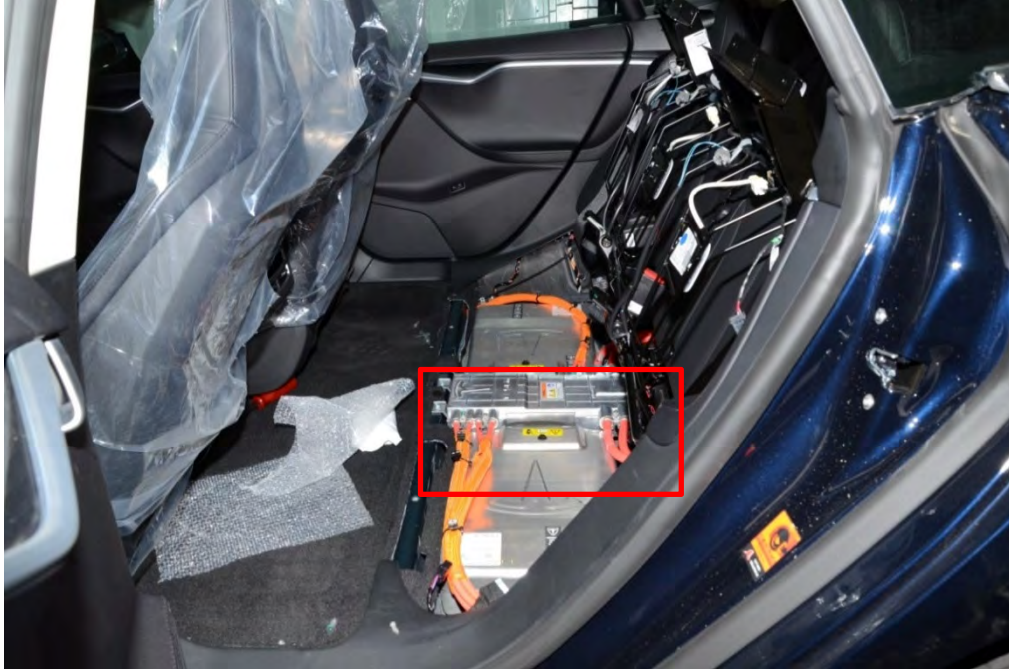
Figure 14 - Manufacturer A vehicle; the DC junction box beneath the rear seat with orange high voltage cables.
