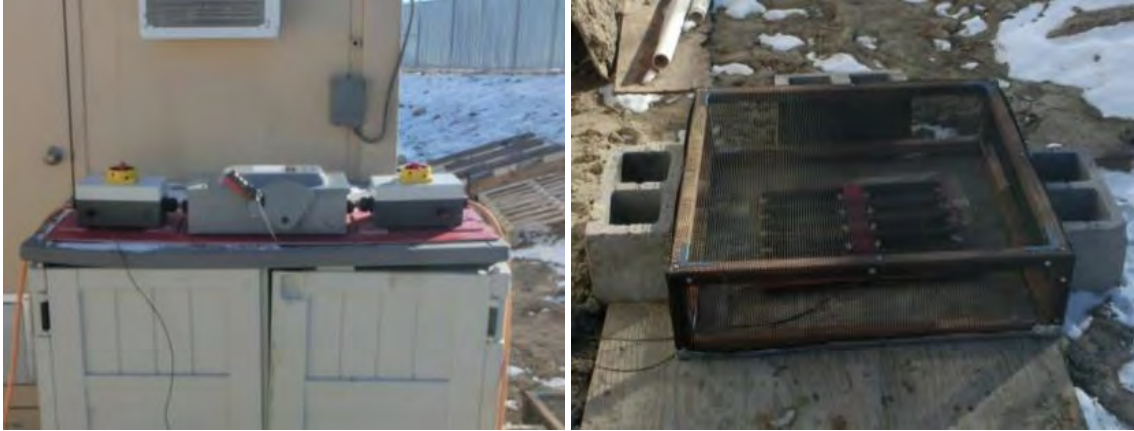
Figure 3 - The switchboard (left) and discharge resistor (right). The discharge resistor is protected beneath a mesh cage to prevent inadvertent contact by an operator. During use, a fan provided cooling air across the resistors to maintain temperature.
