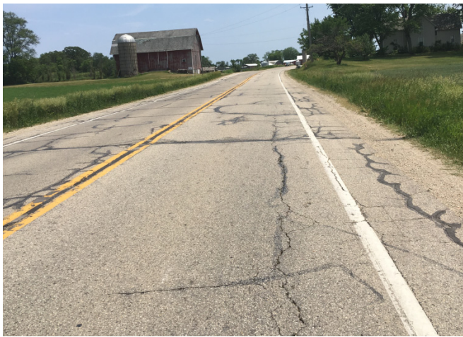
c) Pavement surface distresses
