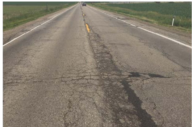
(h) Fatigue cracking
