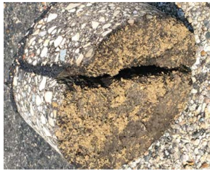
(e) Core from distressed area
