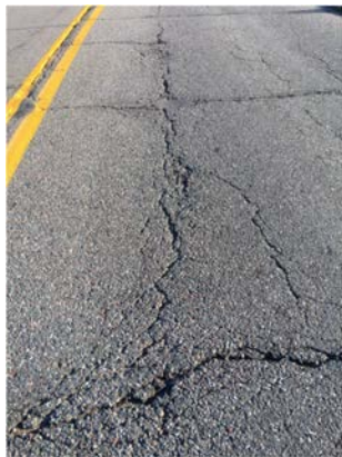
(g) Fatigue cracking
