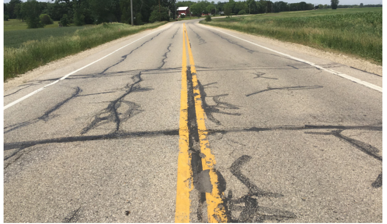
b) Pavement surface distresses
