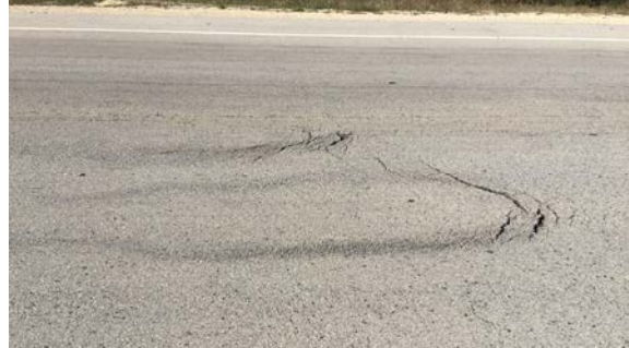
(b) Delamination (slippage)
