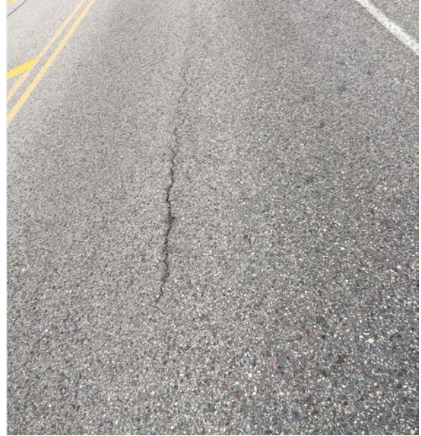
b) Pavement surface distresses
