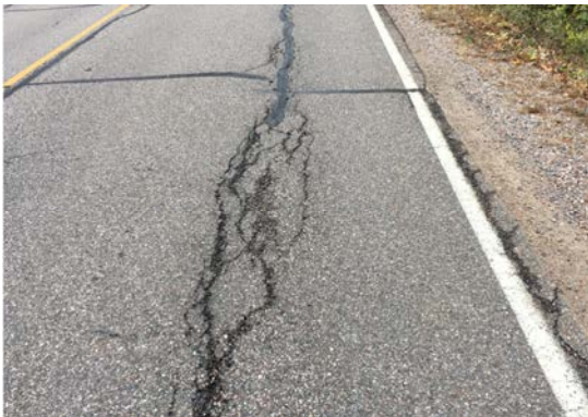
(e) Fatigue cracking and transverse cracking
