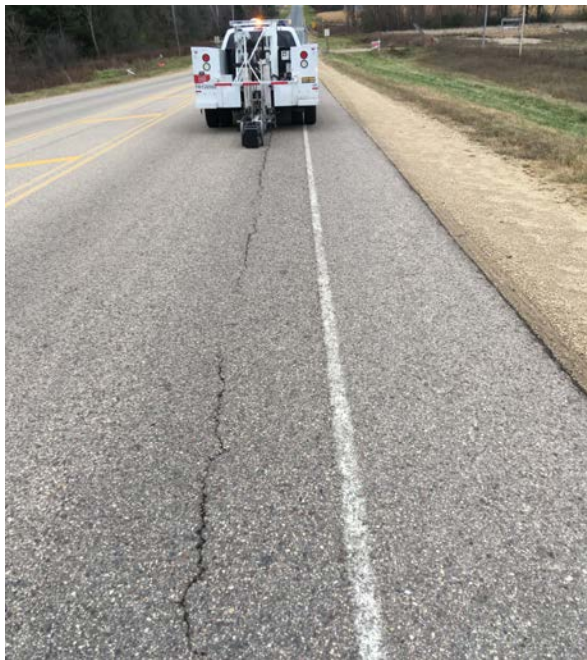
c) Pavement surface distresses
