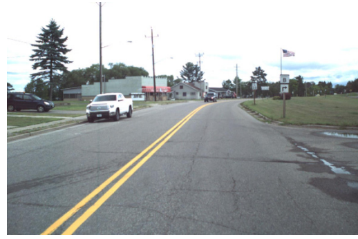
b) Pavement surface distresses
