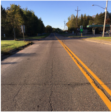
c) Pavement surface distresses
