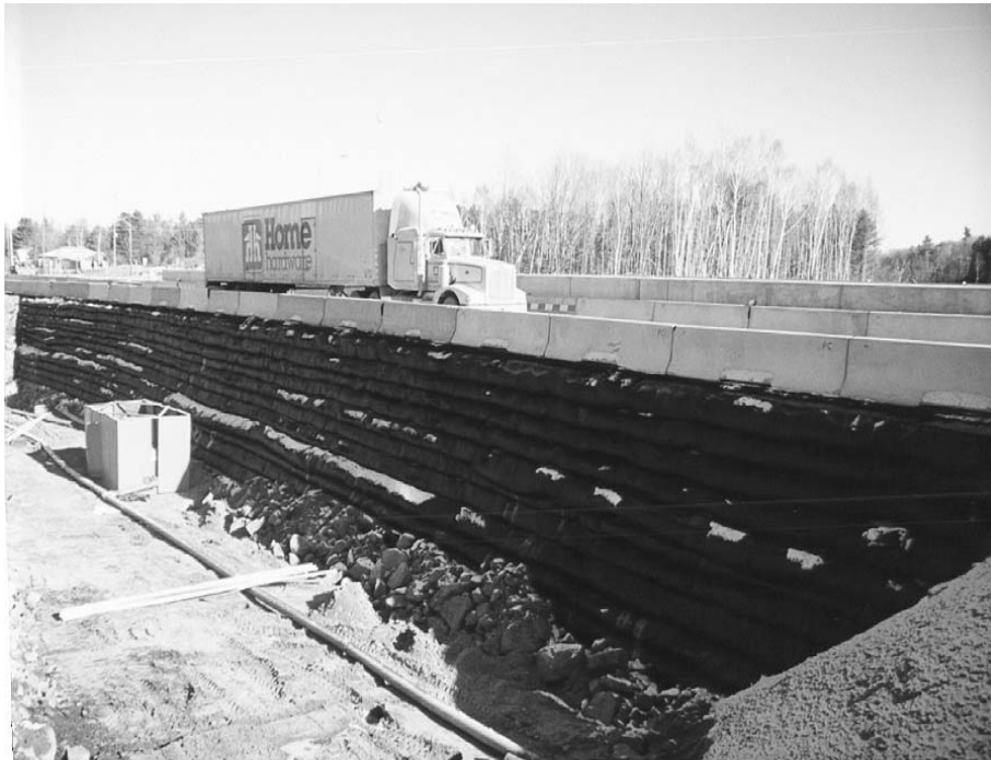
Figure 2-3. MSE wall used to temporarily support a permanent roadway embankment for phased construction.
