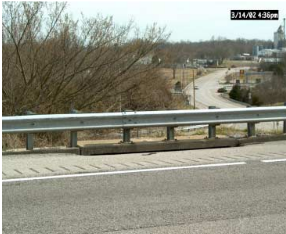
Figure 6. Looking east at KY 255 where the sinkhole is located from I-65 south.
