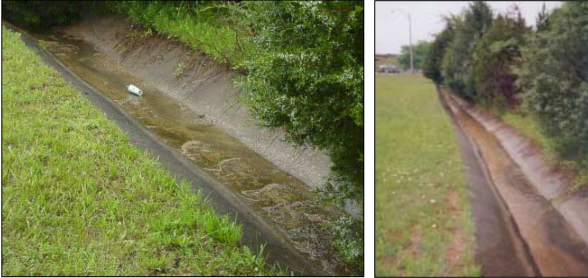
Figure 12. Concrete-lined channel carrying runoff north of KY 255.
