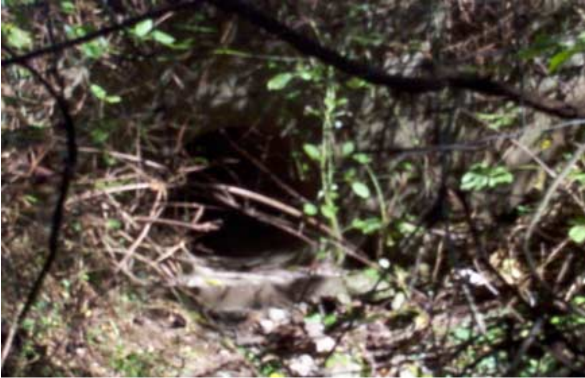
Figure 18. Drain across KY 255 feeding into the sinkhole.
