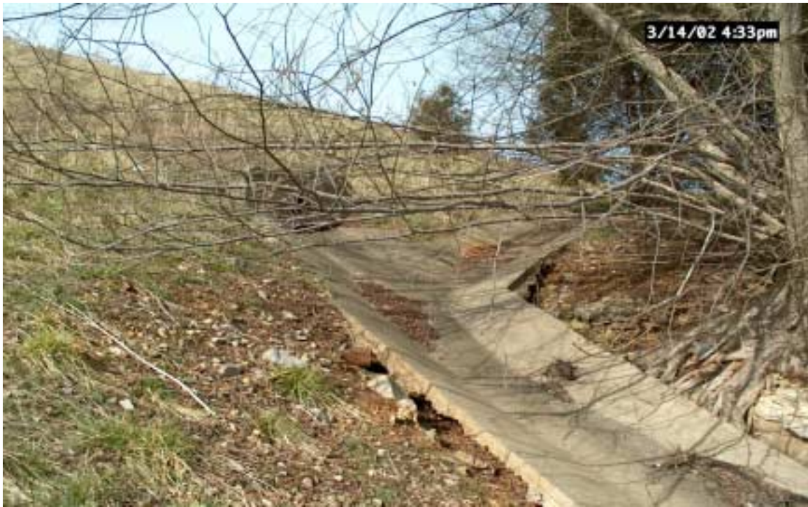
Figure 20. Concrete channel feeding runoff from I-65 N onto north of KY 255.
