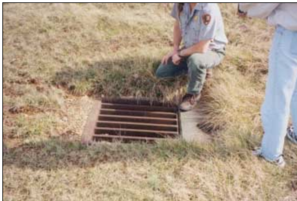
Figure 7. Drainage grates in grassed highway median.
