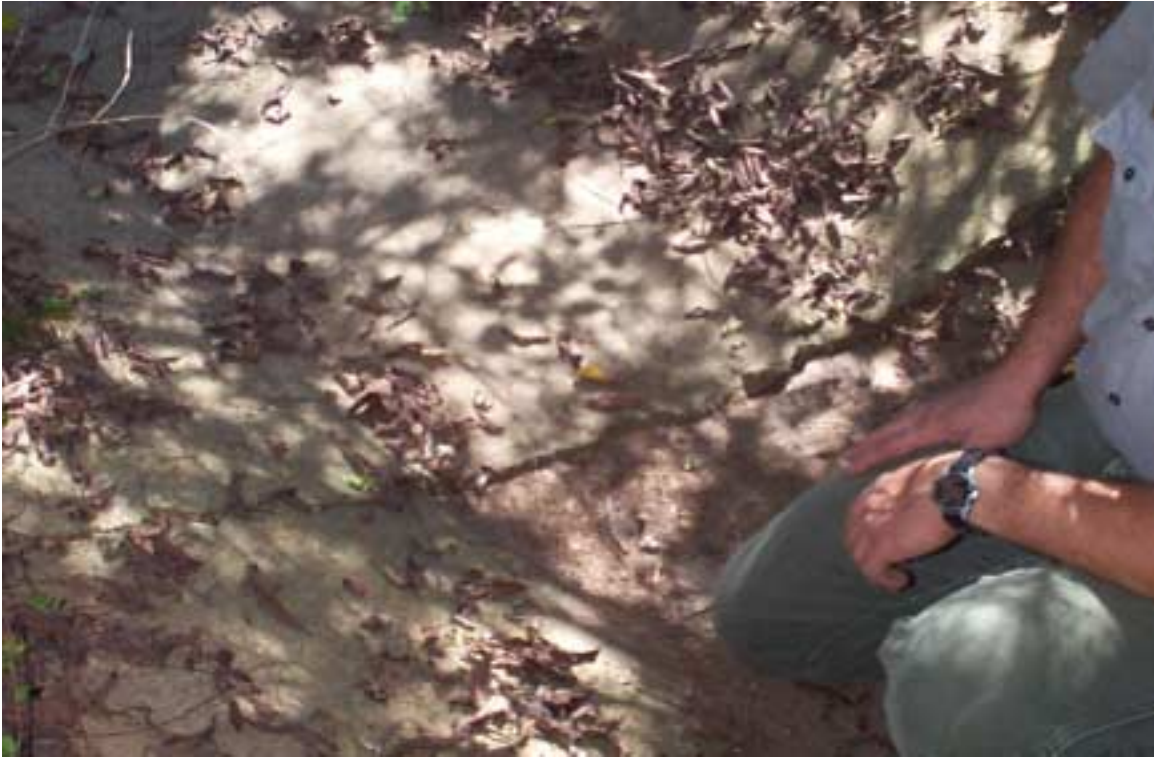
Figure 14. Cracks in the lined channel carrying runoff from I-65.
