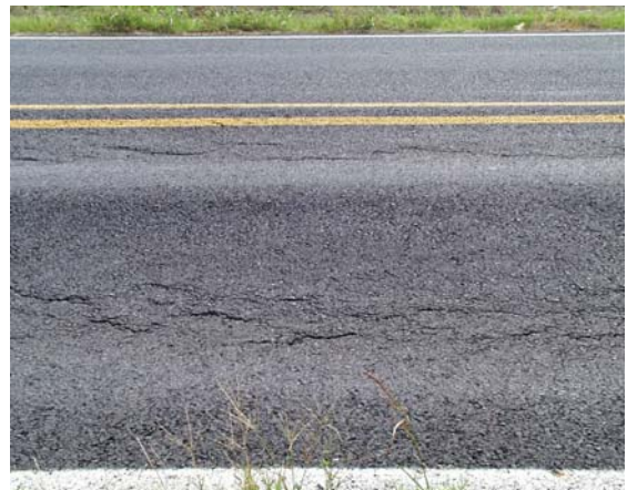
Figure 3.17 Severely fatigued pavement at Hope site
