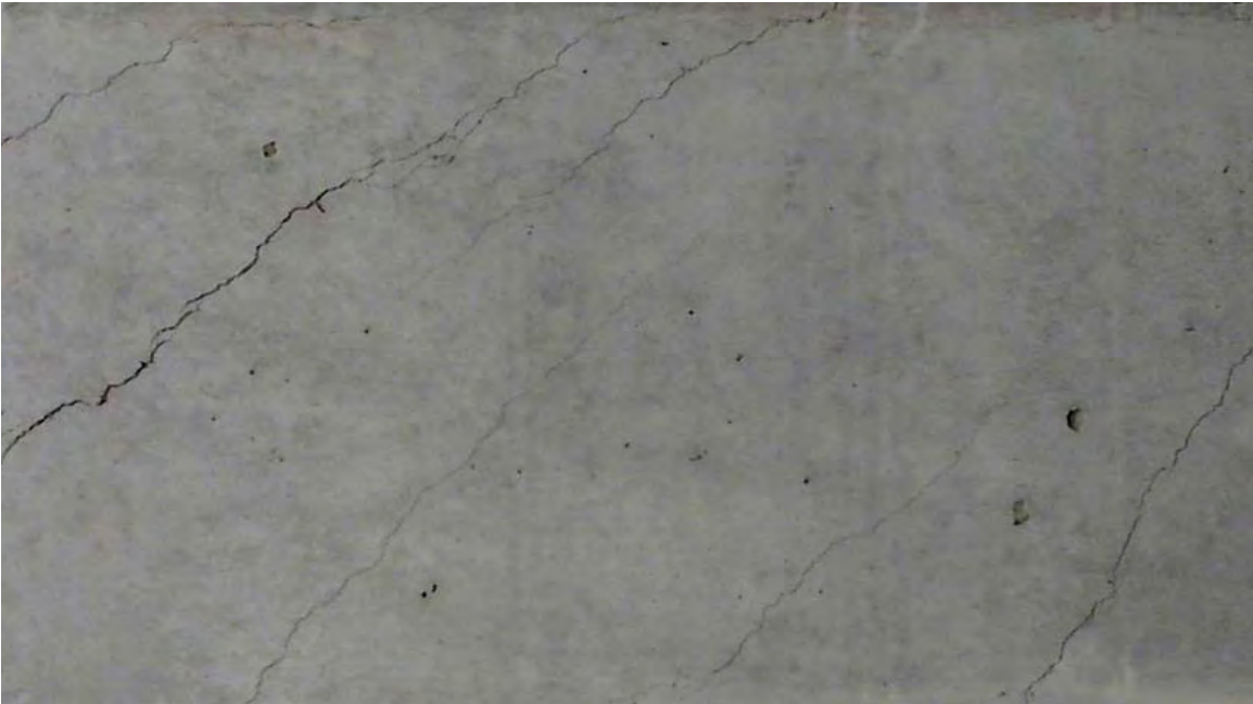
(a) RGB Image of Shear Cracks
