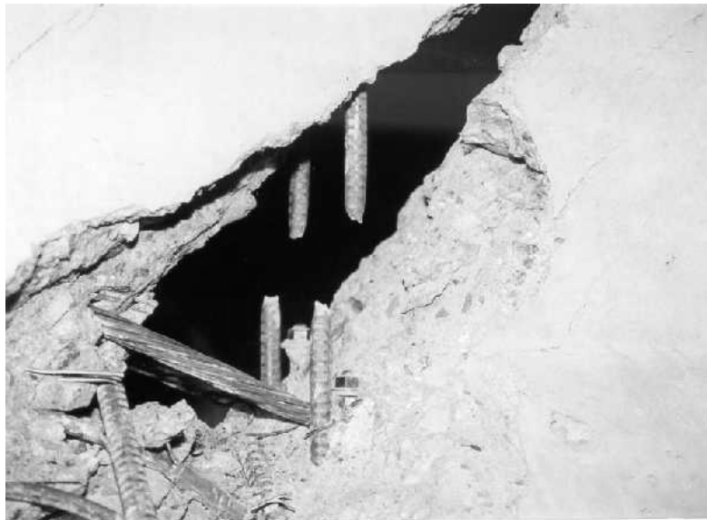
Figure 8.5 Detail of Second End Region Stirrup Failure in the WNEP Beam
