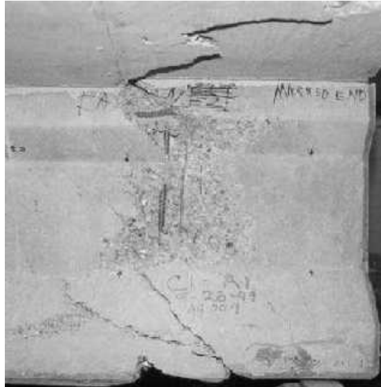
Figure 7.5 Compression Strut Failure of the TNRFf Specimen
