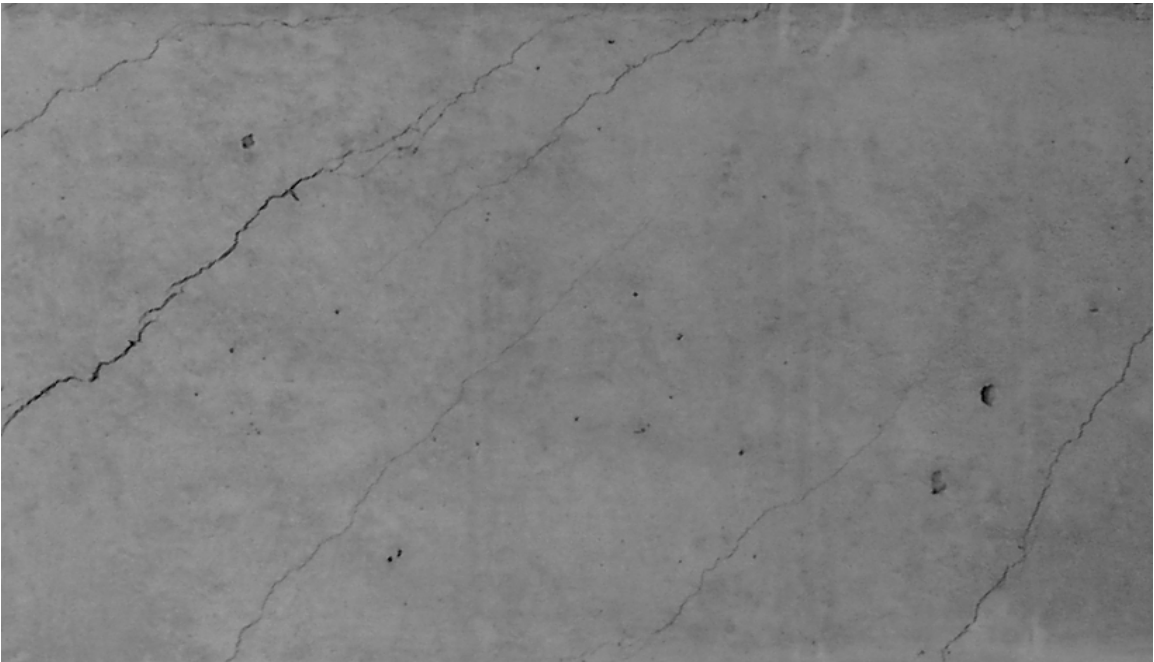
(b) Corresponding Grayscale Image of Shear Cracks
