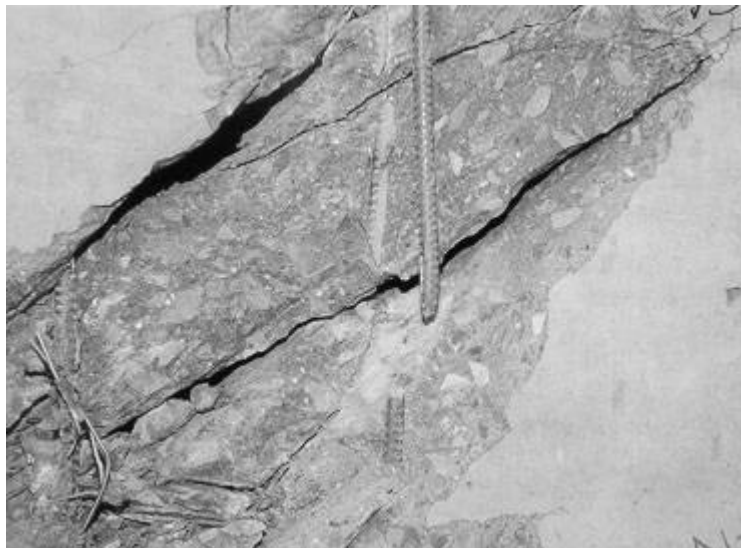
(b) Detail of the Stirrup Failure
