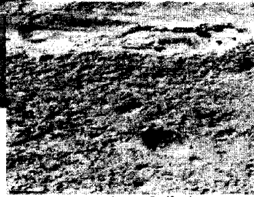
Internal corrosion of oil pipe
