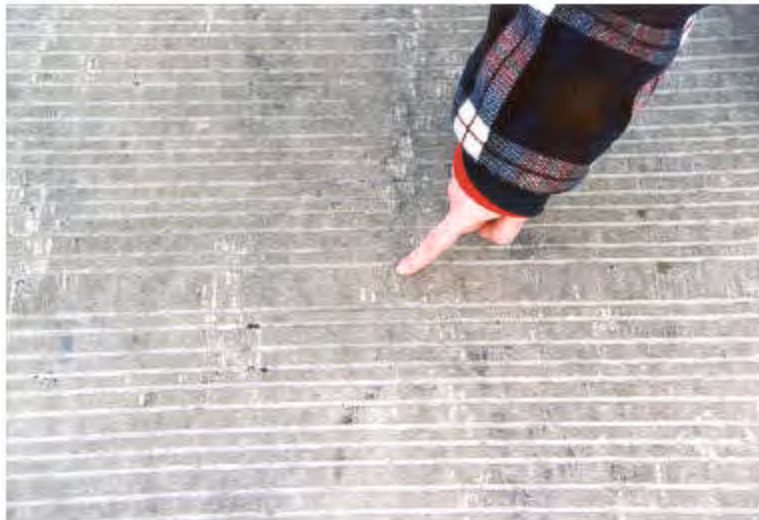
Photo 15. Longitudinal Crack (District 8 – Stage 1, Dec. 1, 1999)
