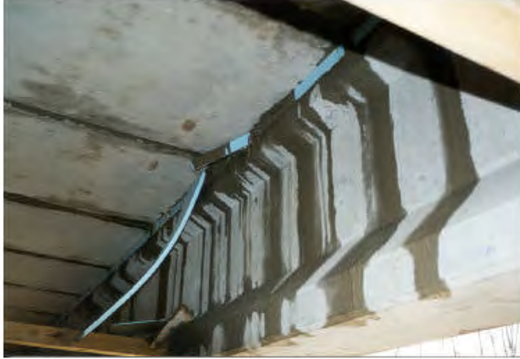
Photo 14. Blowouts (District 6 – Stage 2, March 13, 2000)
