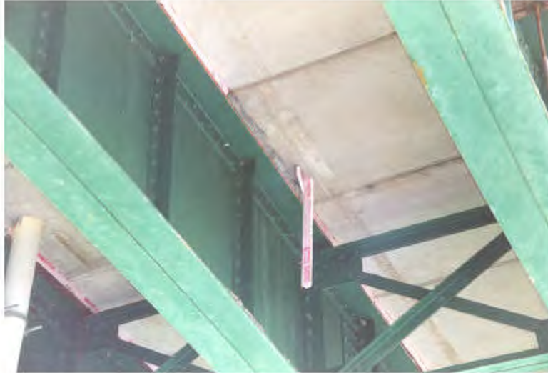
Photo 12. Blowout (District 8 - Stage I, June 28, 1999)
