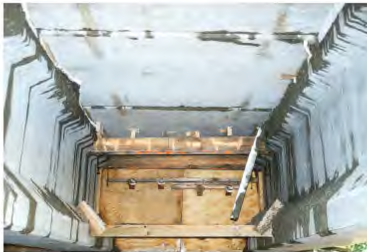
Photo 13. Blowouts (District 6 – Stage 1, August 16, 1999)
