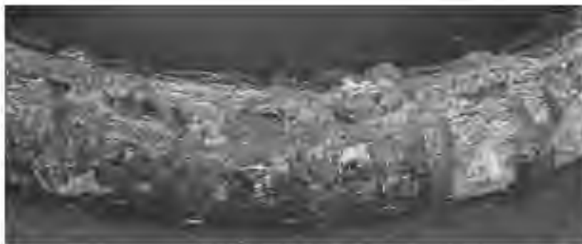
Figure 2.36 Shallow pitting and accumulation of rust products on steel surface under the coating (outside bend).
