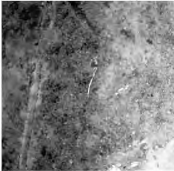
Figure 3.27 Concrete above coated bar.
