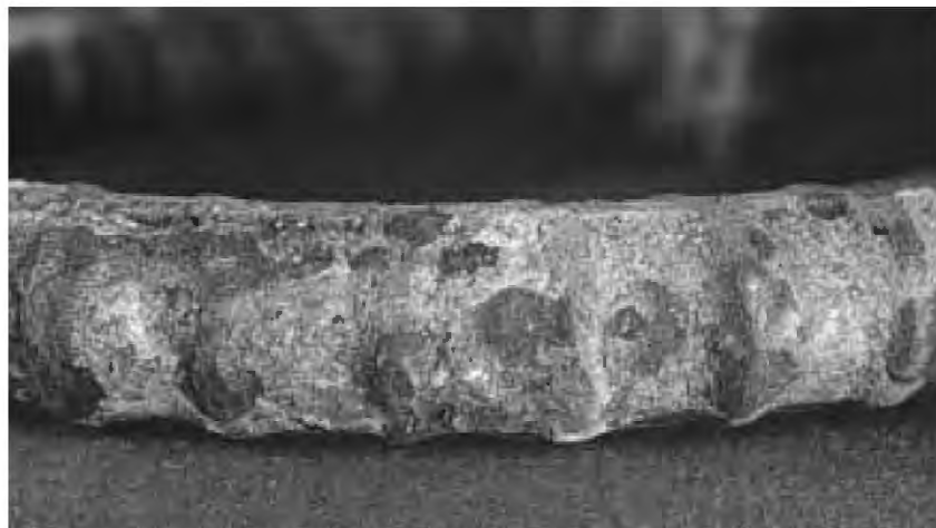
Figure 2.42 Various rust products above uniformly black corroded surface under the coating.
