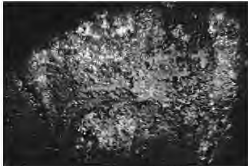
Figure 3.17 Surface corrosion of coated bar after one year of exposure.
