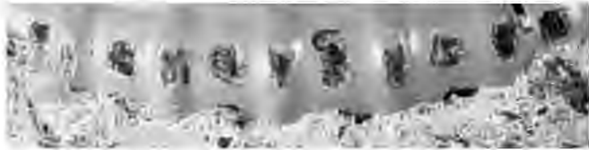
Figure 3.31 Corrosion initiation around exposed steel areas on damaged coated bars embedded in concrete.
