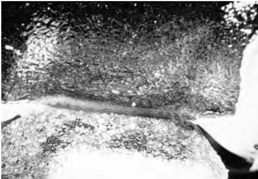
Figure 2.41 Trapped solution beneath epoxy coating.
