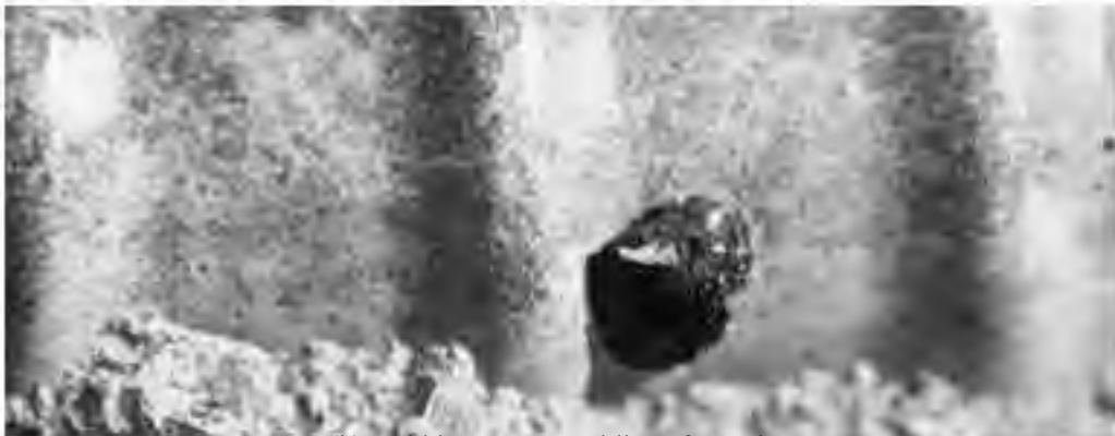
(b) Void in concrete at blister formation
