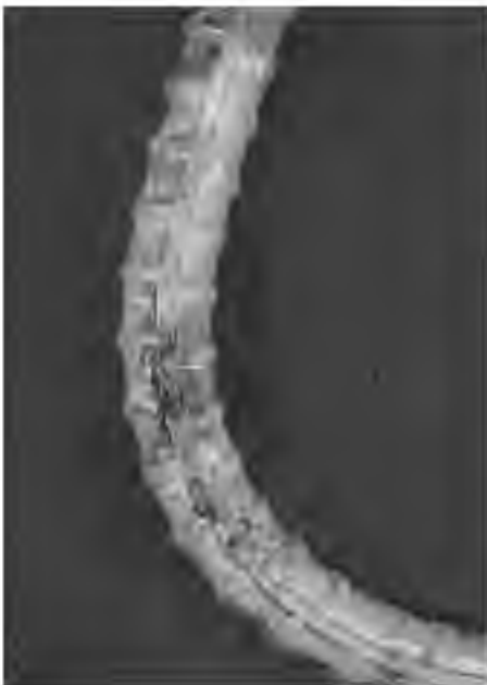
(a) Rust staining and blistering on epoxy-coated bar.
