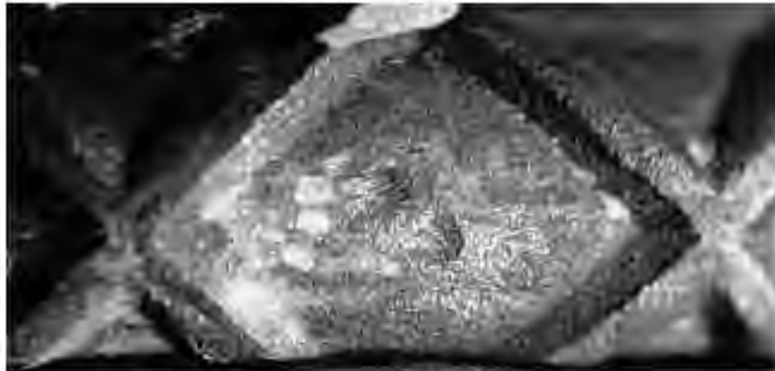
Figure 2.39 Darkening and pitting underneath patching.
