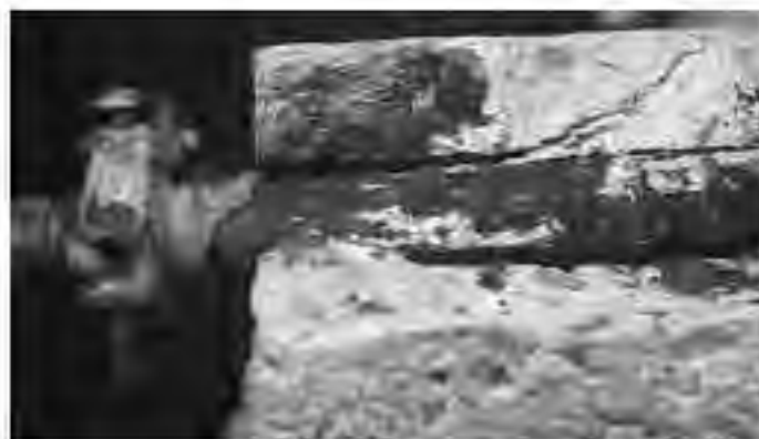
(b) Another aspect of rust inside crack surface.
