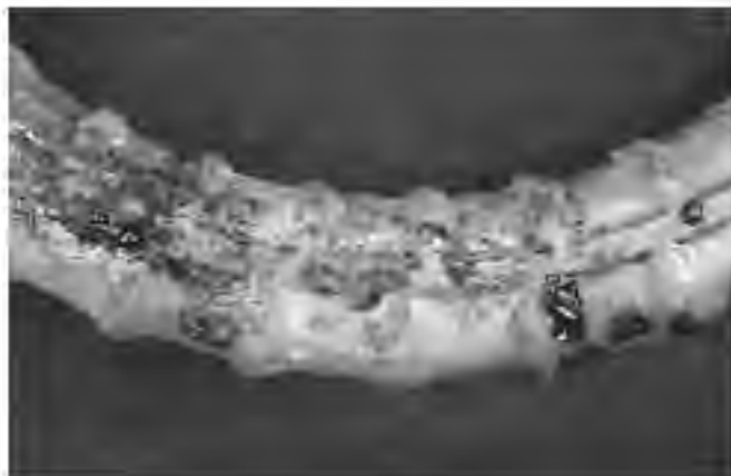
(b) Rust staining and exudation of brown liquid on epoxy-coated bar.
