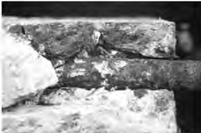
(c) Pitting at straight leg of 25-mm (#8) uncoated bar after 4.5 years of exposure.
