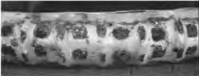
Figure 2.28 Corrosion of damaged areas at outside bend on bar 3B.5.
