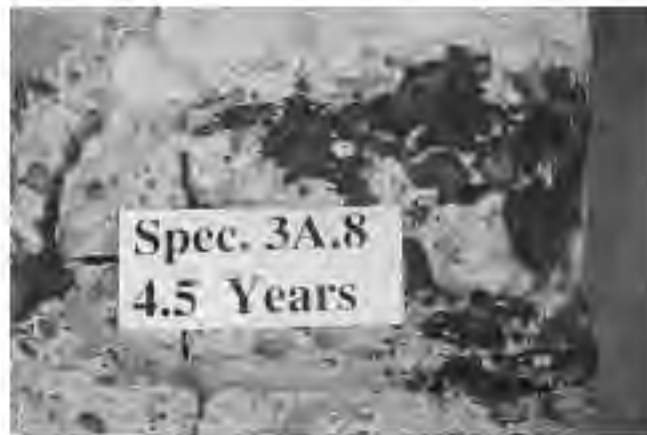
Figure 2.48 Rust staining on surrounding concrete under uncoated bar 3A.8.
