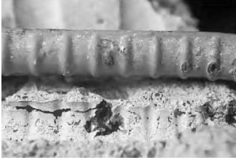
Figure 3.24 Blisters always formed adjacent to concrete voids.
