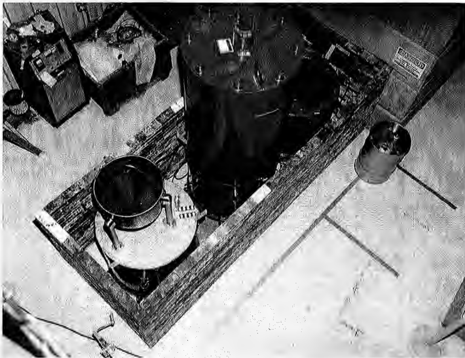
Fig. 17. Photograph showing shielded containers, shielded remote transfer bell, lead brick-shielded area, and remote vermiculite hopper for the CsRD.
