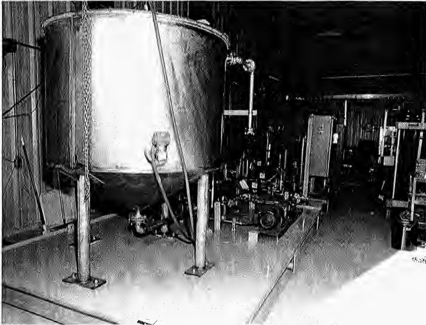
Fig. 12. Photograph of the CsRD feed tank skid with no shielding.
