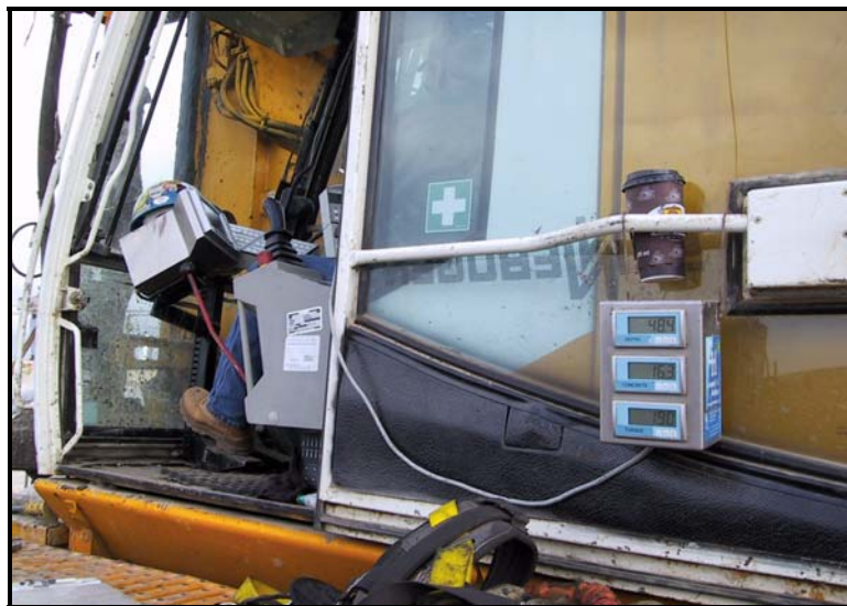
Figure 7.5: Display Panel for Observation by Inspector
