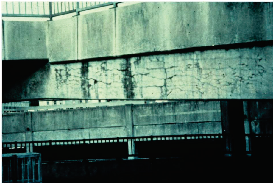
Figure 4 – Aligned cracking in beam (Condition State 3)
