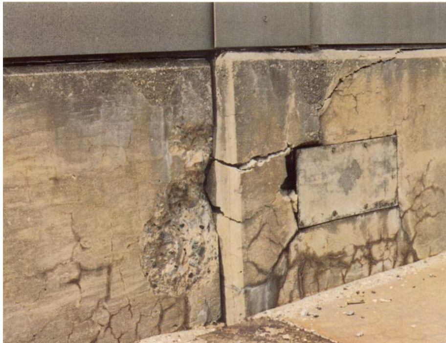
Figure 6 – Relative dislocation/misalignment, leading to loss of clearance and cracking (photo from SHRP C-315, 1991) (Condition State 3)
