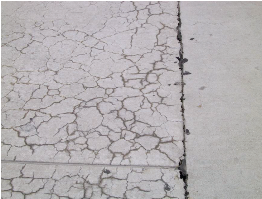
Figure 8 – Joint Sealant Failure in Concrete Pavement (Condition State 3)
