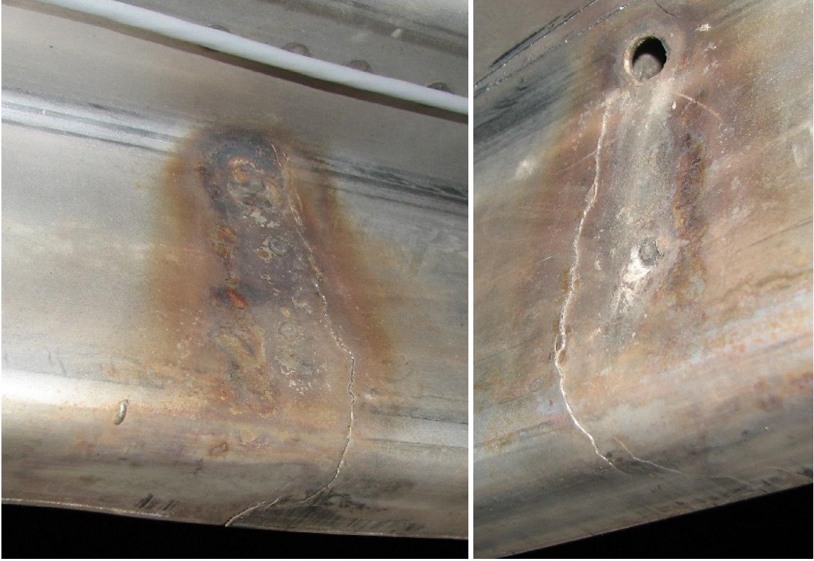
Figure 20. Cracks in Right Side Sill
