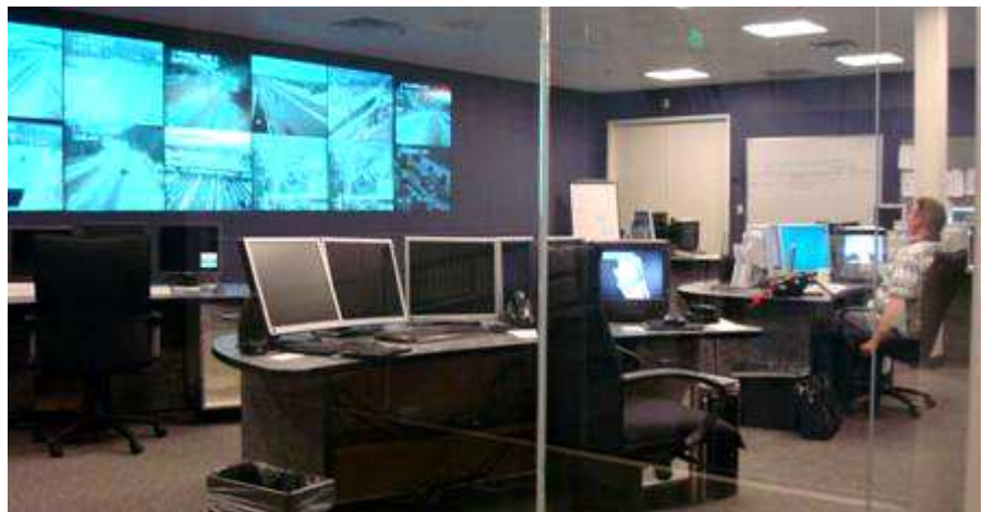
Exhibit A8 – CTMC Control Room Viewed from Media Room
