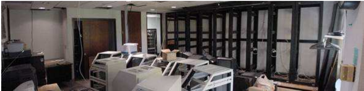
Exhibit 2 – ITOC Operations Room (October 2005)
