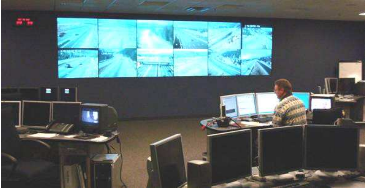
Exhibit 6 – CTMC Operations Room (October 2007)
