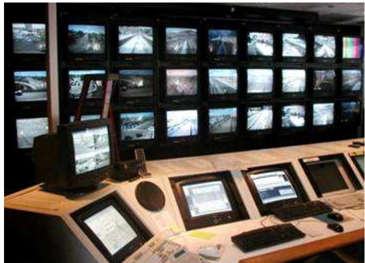
Exhibit 1 – ITOC Operations Room (September 2005)
