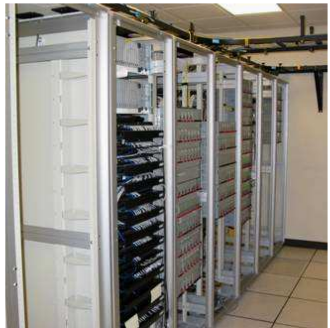
Exhibit A4 – CTMC Computer Room Equipment Racks
