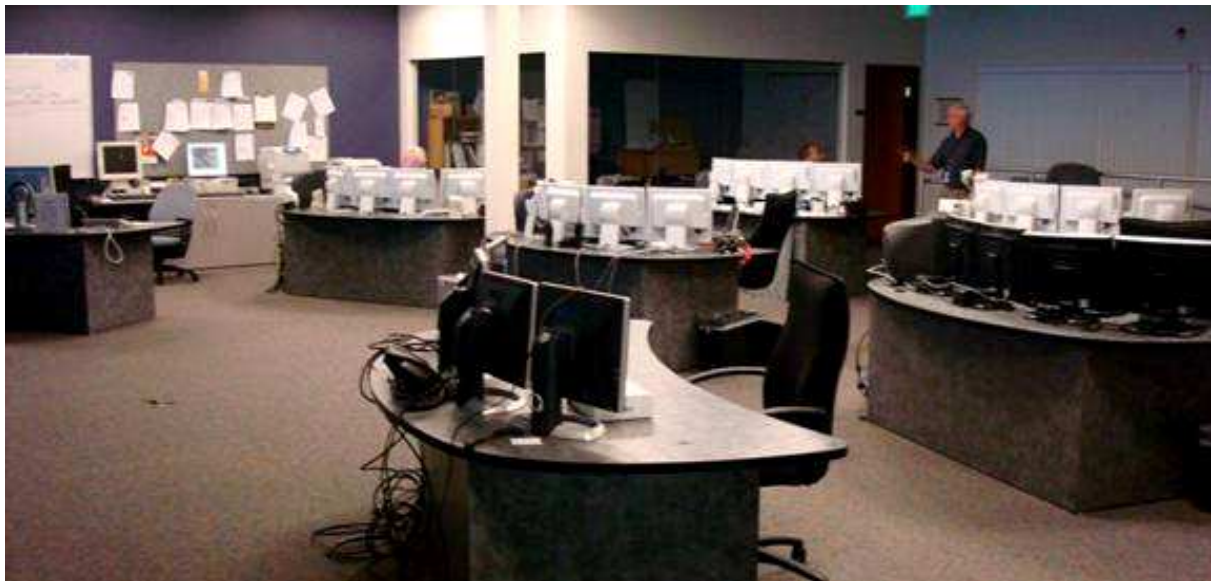
Exhibit 12 – CTMC Control Room
