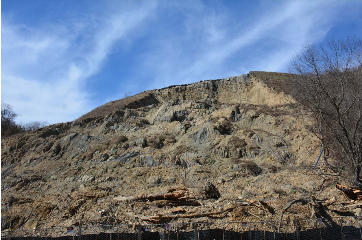
Figure 1-4. Geosynthetic rupture in reinforced tall slope [Yeager Airport, Charleston, WV, March 2015]
