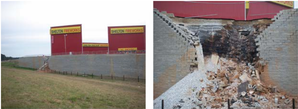
Figure 1-3. Geosynthetic reinforced wall: limit state shallow failure [I-85 near Exit 70, Cusseta, Alabama; photo taken February 2007]
