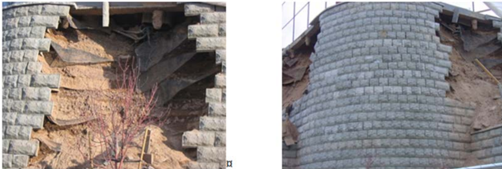
Figure 1-1. Result of missing reinforcement: close-up (left) and general view (right) [January 2008, Salt Lake City, Utah]
