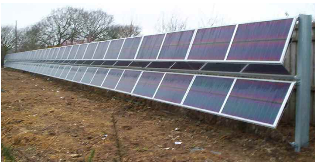
Figure 9. Completed installation of the solar modules at the top of the slope
