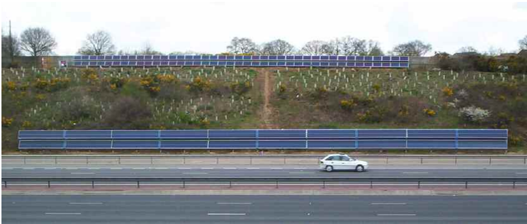
Figure 10. Completed installation as viewed from the opposite side of the M27 motorway
