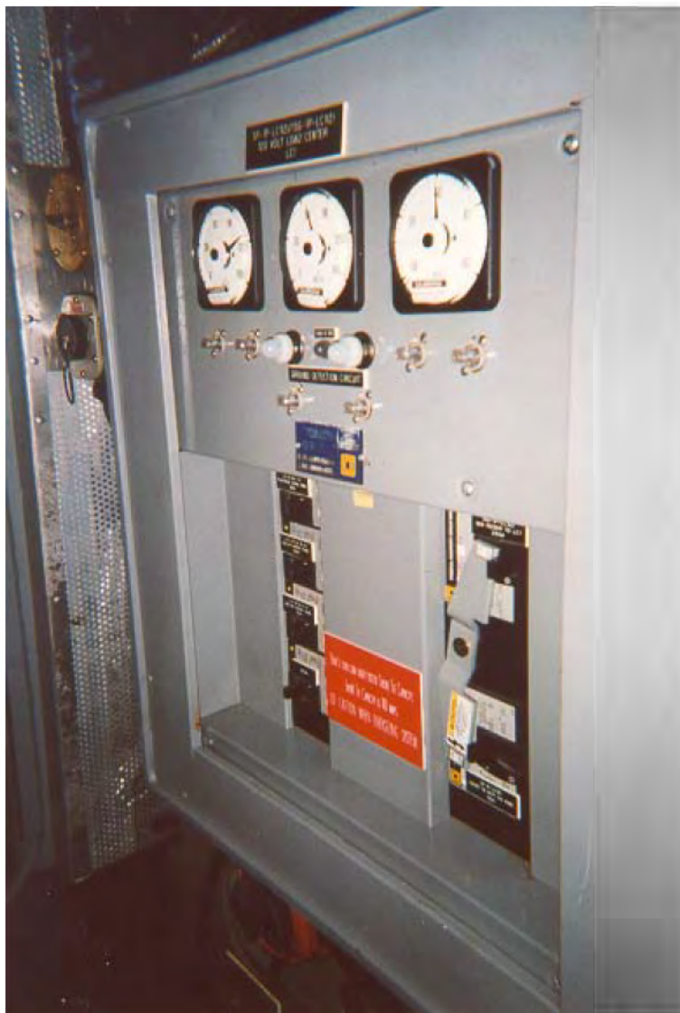
Figure 3-21 120-VAC Load Center (LC) 1
