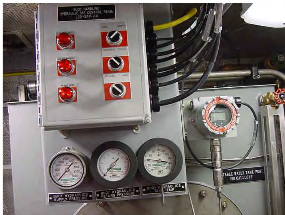
Figure 3-36 Buoy Handling Hydraulic System Control Panel (Machinery Space)
