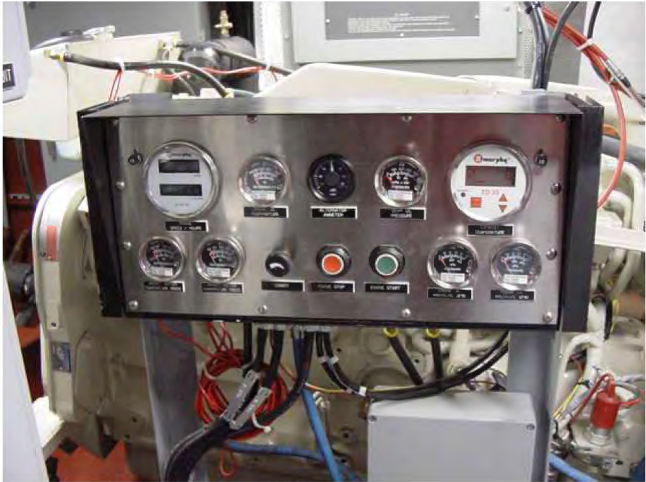
Figure 3-6 Engine Control and Gauge Panel - Machinery Space
