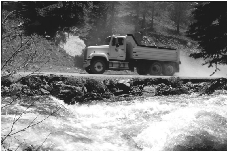
Figure 33. Erosion of fillslope and side-cast material by Geneva Creek, high streamflow, June 1995.
