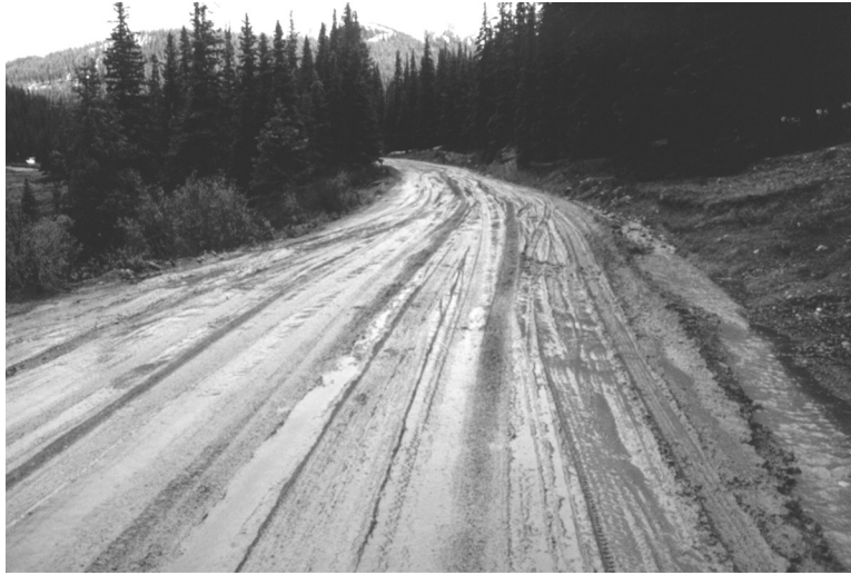
Figure 36. Rutting and erosion of the road surface just south of Naylor Creek.
