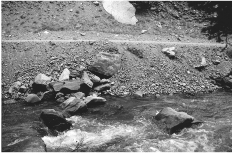
Figure 34. Appearance of fillslope at low streamflow in Geneva Creek after repair and regrading of road, August 1995.
