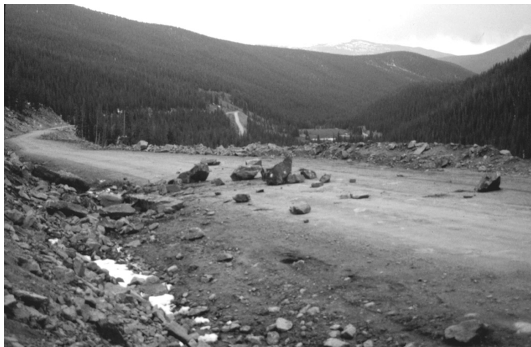
Figure 29. Boulders eroded from cutslope on Guanella Pass road near disused ski area, May 1996.
