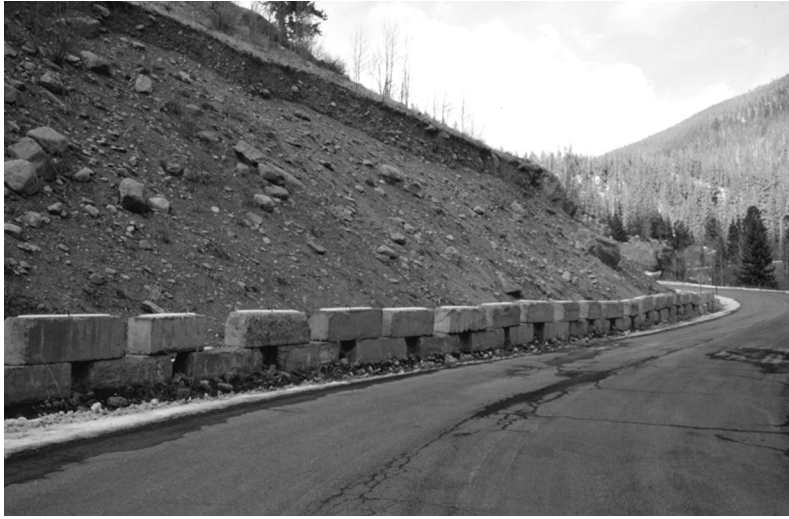
Figure 32. Cutslope along Guanella Pass road in the Falls Hill segment just north of the Scott Gomer Creek crossing, January 1994.
