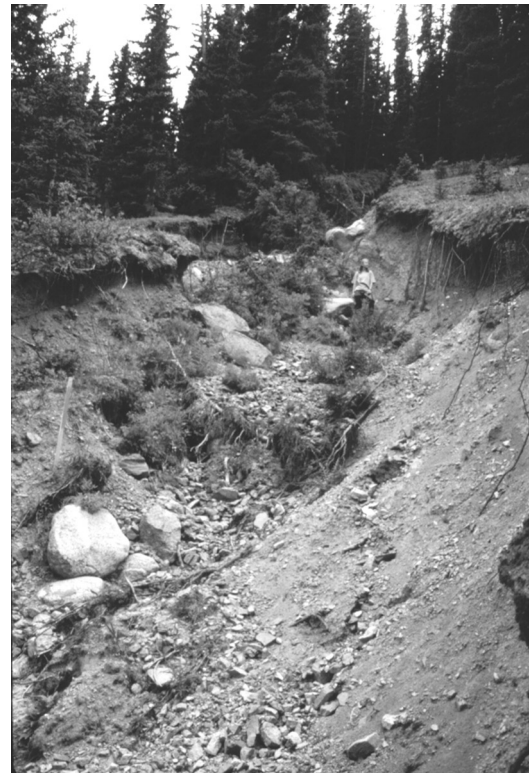
Figure 38. Eroded road-runoff channel about 200 feet below the Guanella Pass road, located in the switchback road segment south of Naylor Creek, August 1996.
