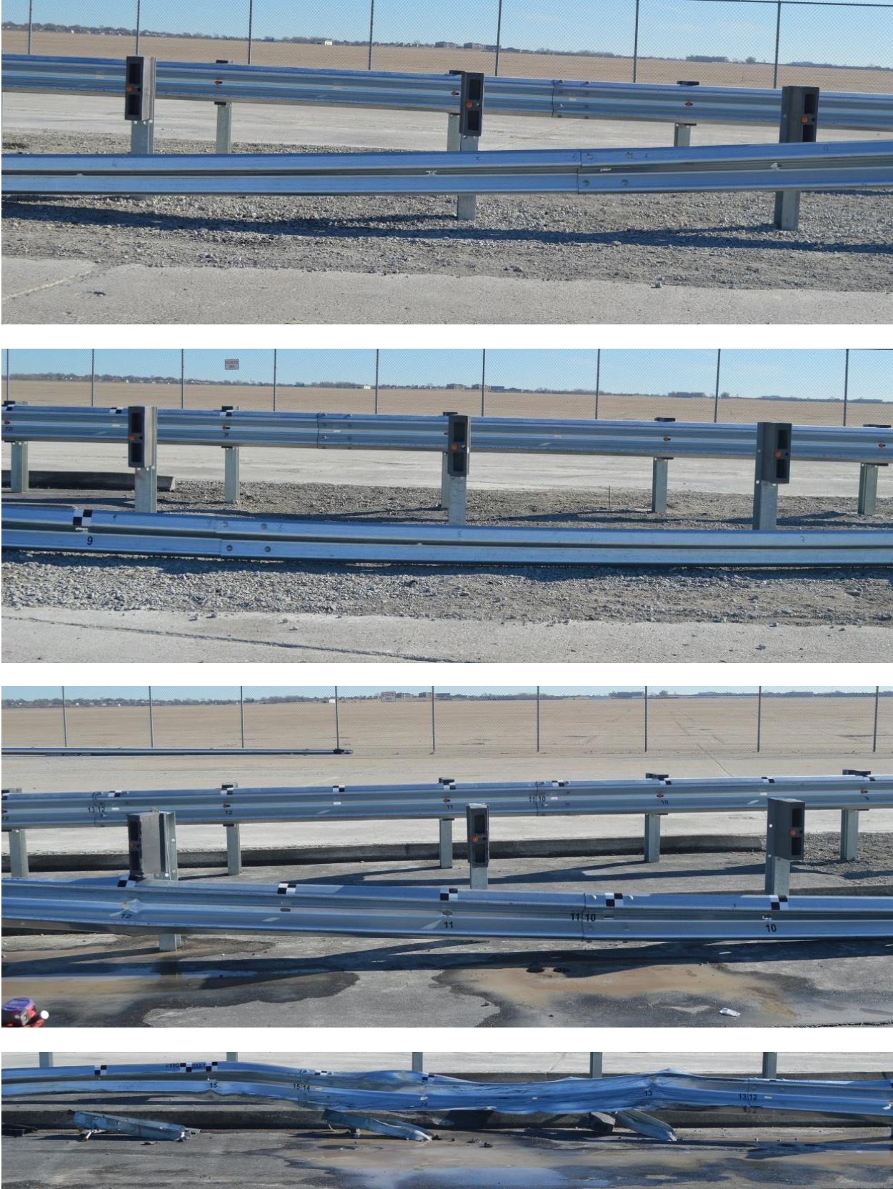
Figure 38. System Damage – Post Nos. 4 through 15, Test No. GAA-1
