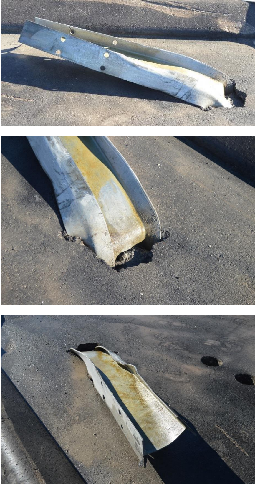
Figure 42. Post No. 14 Damage, Test No. GAA-1
