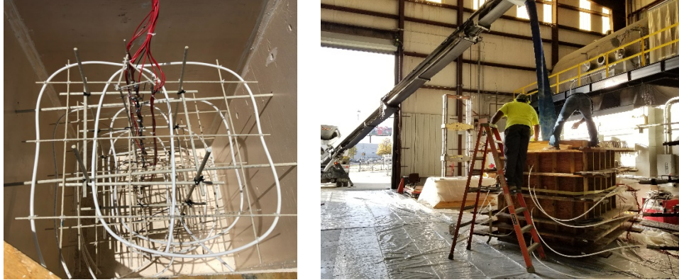
Figure 13. The inside frame (left) and the cooling pipes (right)
