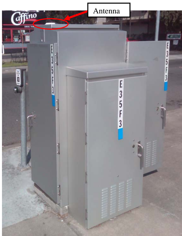
Figure 4. Antenna Mounted on Top of Controller Cabinet (White Dish on Left-hand Side).
