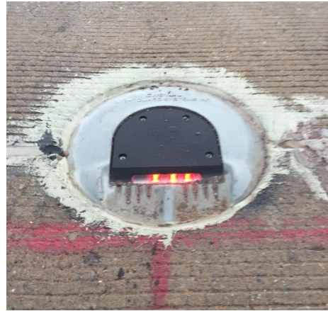
Figure 14 – Light with Burned out LEDs
