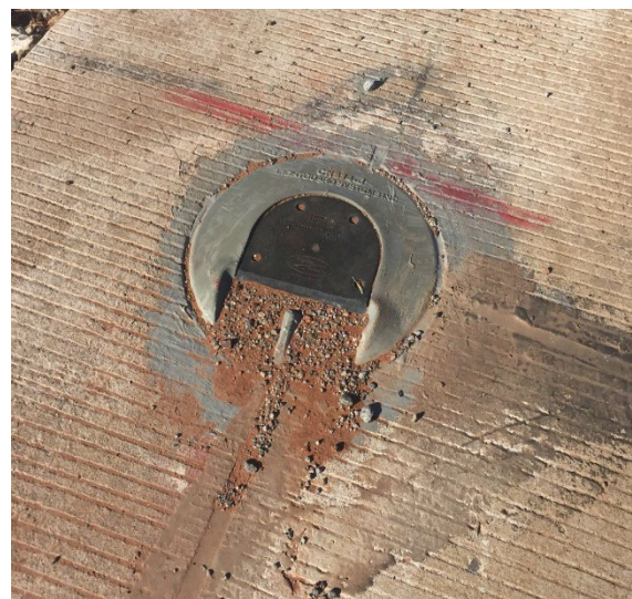
Figure 13 – Example of dirt accumulating on in-pavement light fixture
