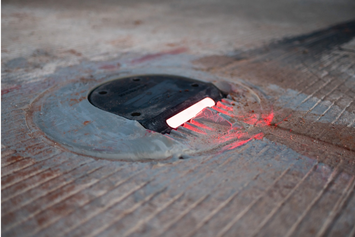
Figure 4 – Close-up of in-pavement light fixture in Elk City
