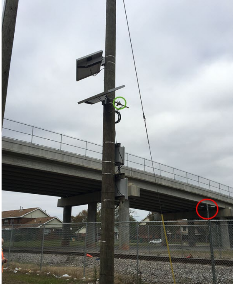
Figure 10. Post Construction Video Data Collection Systems in Collegeville, AL
