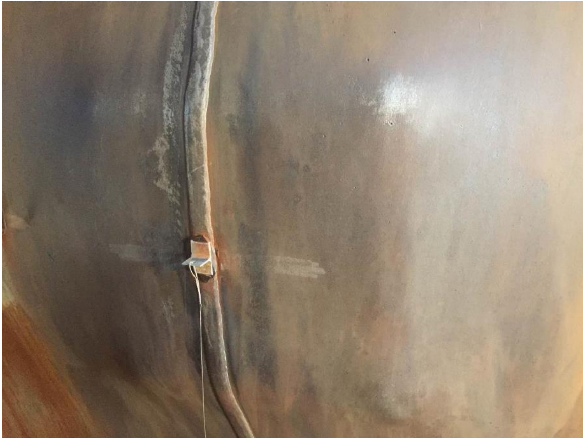
Figure 20. Interior of Impact Zone, Post-Test
