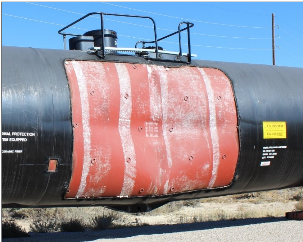
Figure 19. Tank Car Indentation—After Removing Jacket and Insulation Section
