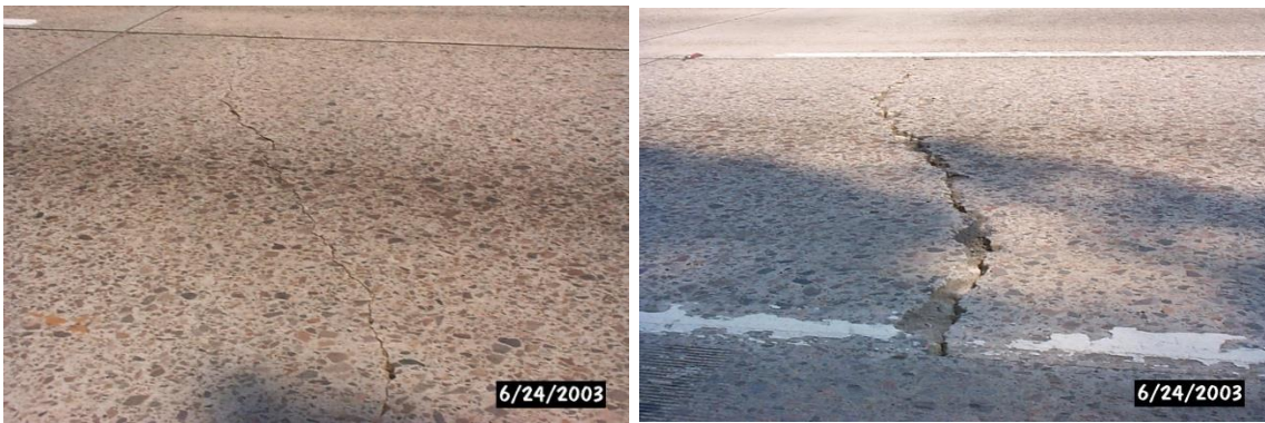
Figures 4-5 Example of transverse cracking, Severity Levels 1 and 2
