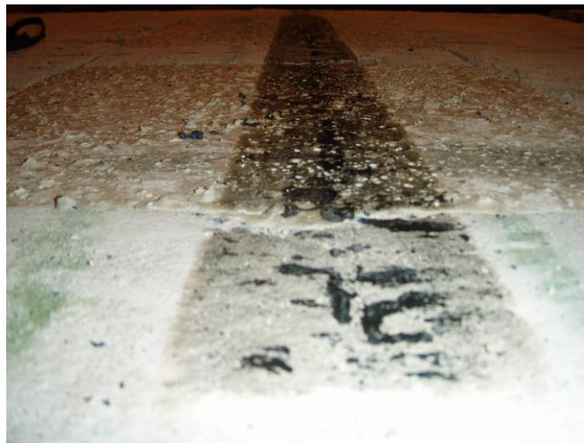
Figure B-14: Rapid Set Patch after Tire Load Simulation – Close-up 3
