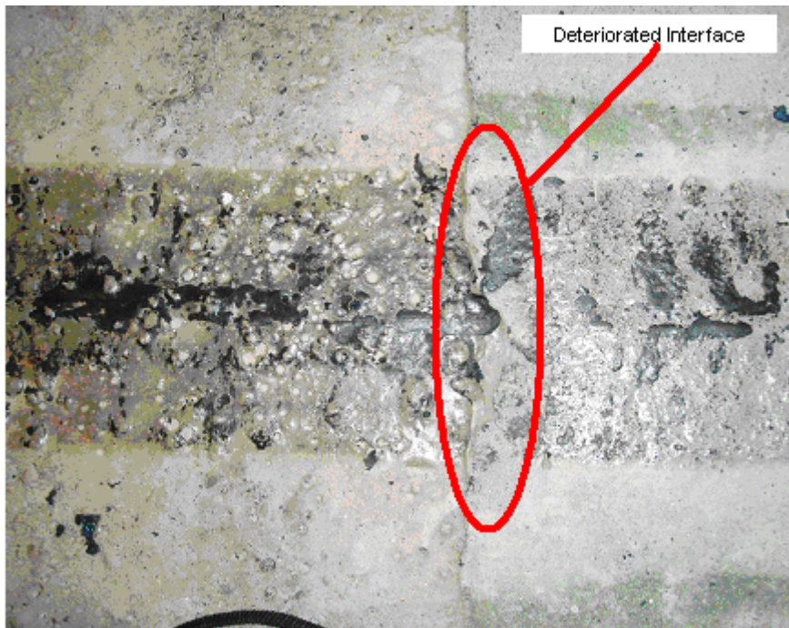
Figure 3-27: Repetitive Tire Loading – Rapid Set Patches – Deteriorated Interface
