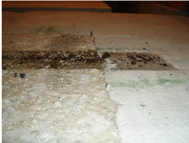
Figure B-13: Rapid Set Patch after Tire Load Simulation – Close-up 2
