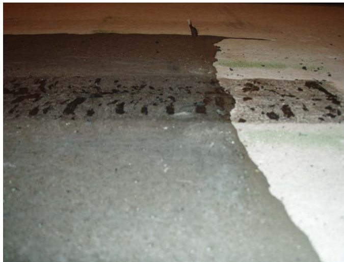
Figure B-10: Pavemend 15.0 Patch after Tire Load Simulation – Close-up 2
