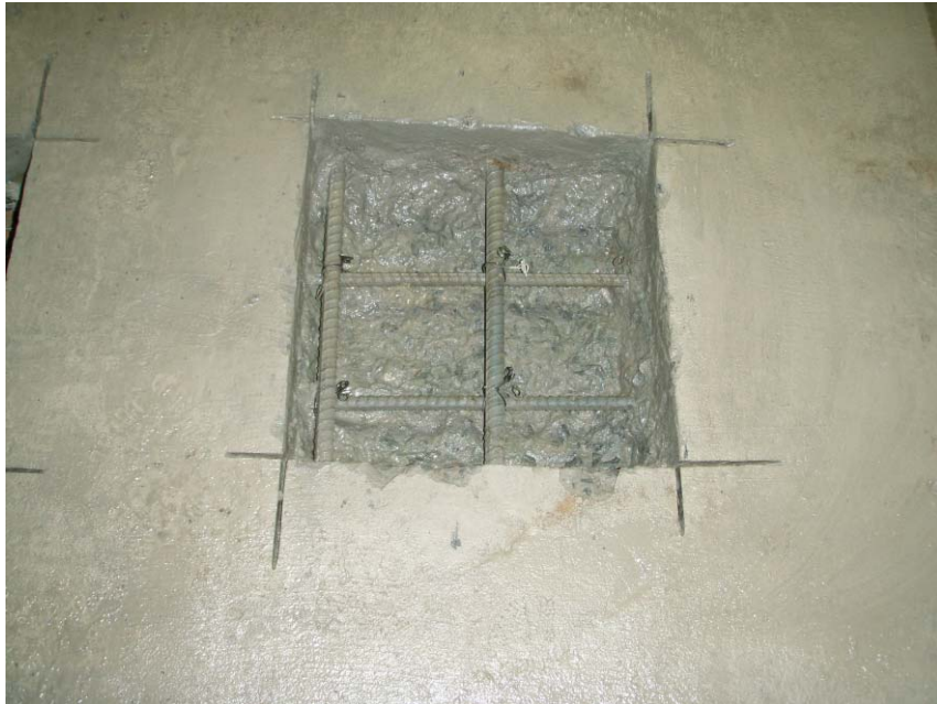
Figure 3-7: Jackhammered Patch Area – Half Depth
