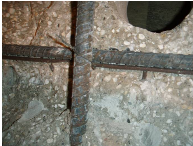
Figure 3-48: Rapid Set Corrosion Slab – Close-Up 2
