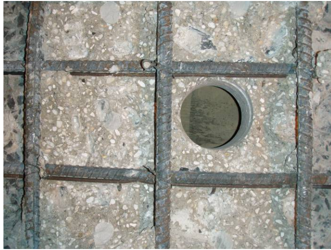
Figure 3-47: Rapid Set Corrosion Slab – Close-Up 1
