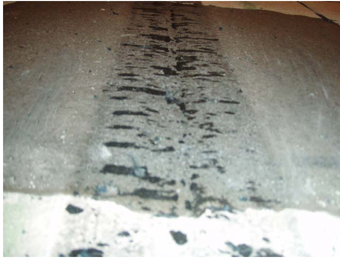
Figure B-11 : Pavemend 15.0 Patch after Tire Load Simulation – Close-up 3
