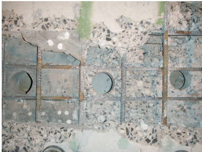
Figure 3-46: Pavemend 15.0 Corrosion Slab – Close-Up 2
