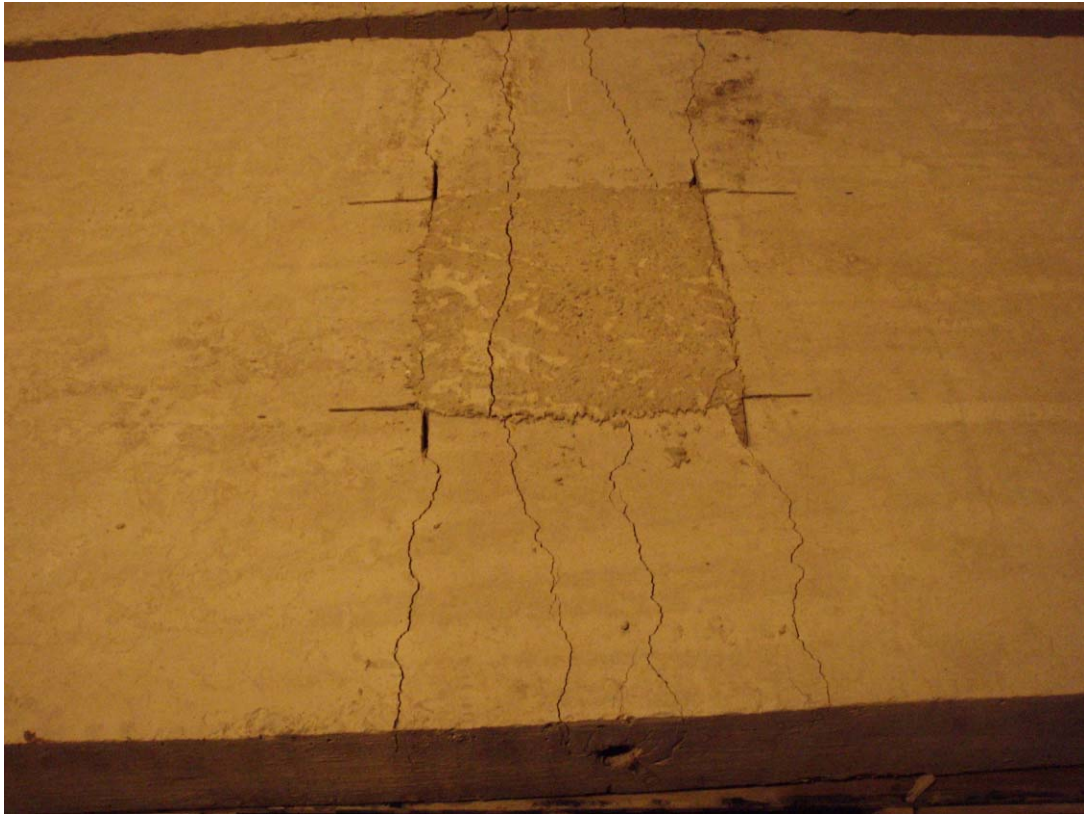
Figure 3-20: Cracking of Rapid Set Slab
