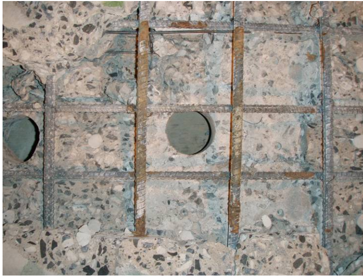
Figure 3-45: Pavemend 15.0 Corrosion Slab – Close-Up 1
