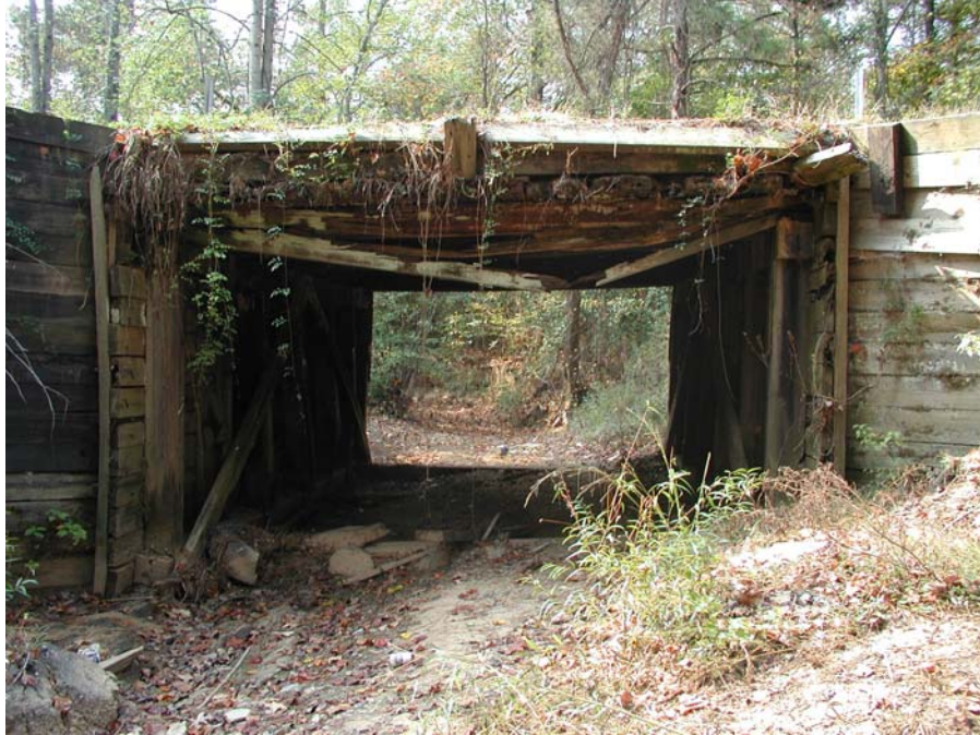
Figure 2-1. Timber structure showing signs of distress
