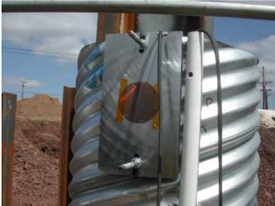
Figure 30. Soil pressure gage (41)
