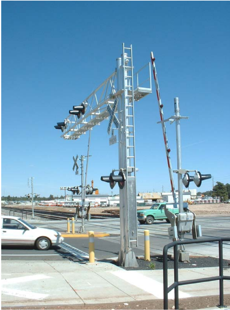
Figure 3: Photo Of At-Grade Crossing Equipment At The Study Site
