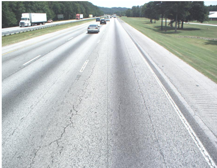
FIGURE I.6: Pavement Conditions of Test Site #3
