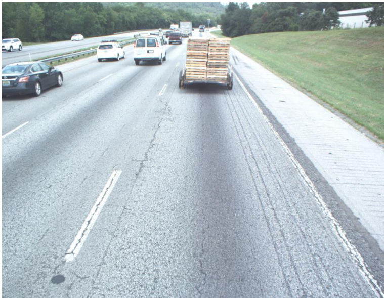
FIGURE I.8: Pavement Conditions of Test Site #4
