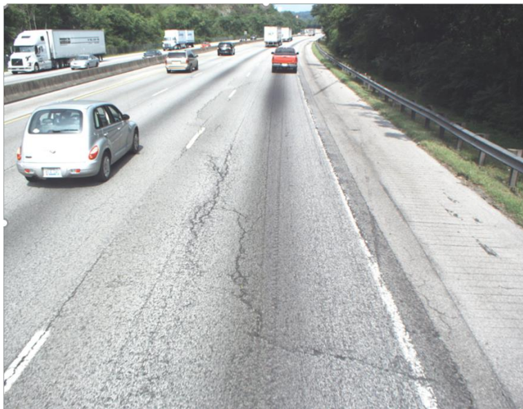
FIGURE I.2: Pavement Conditions of Test Site #1
