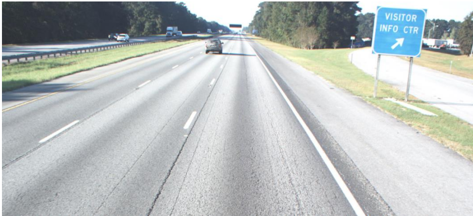
FIGURE I.20: Pavement Conditions of Test Site #7
