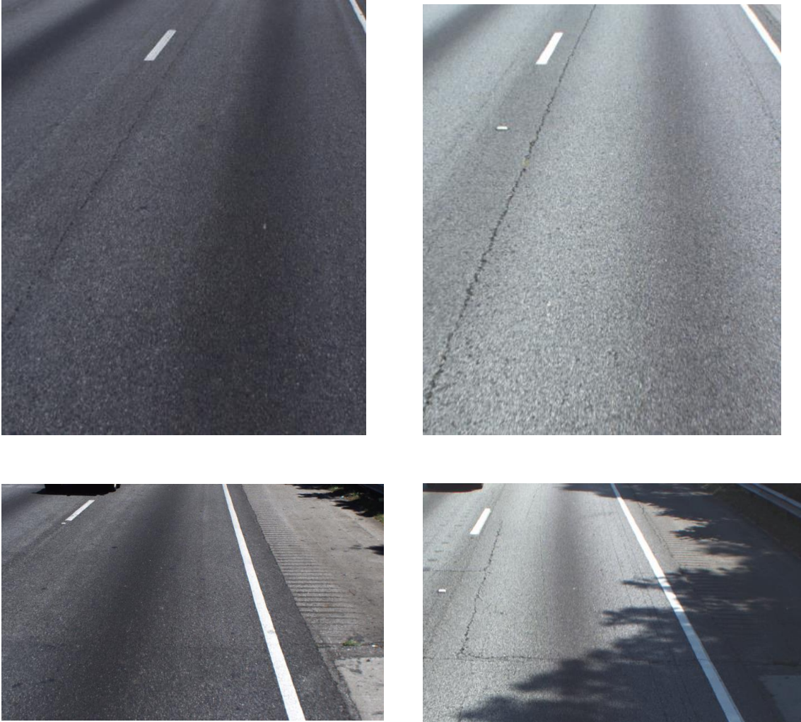
FIGURE 11: Examples of Cracking on I-285 in 2013 (Left) and 2017 (Right)
