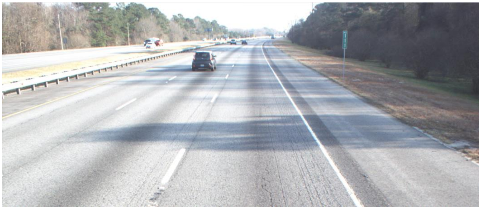
FIGURE I.18: Pavement Conditions of Test Site #6
