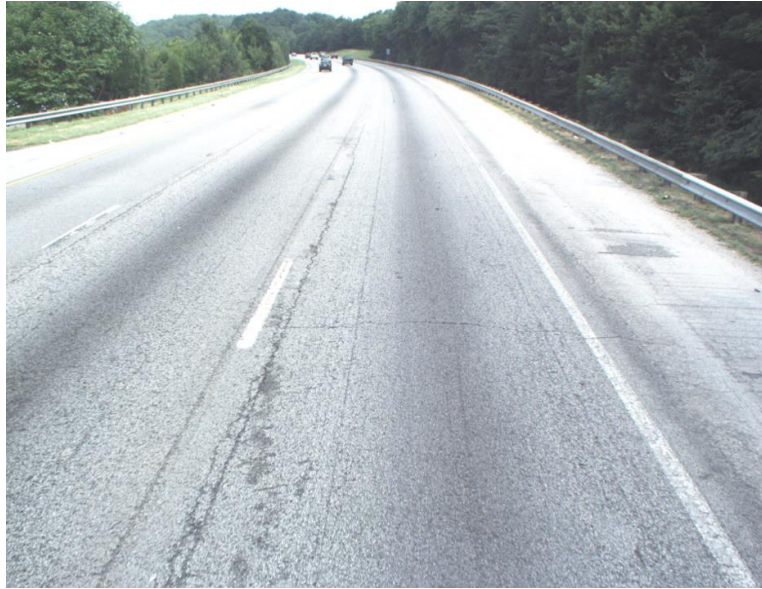
FIGURE I.4: Pavement Conditions of Test Site #2
