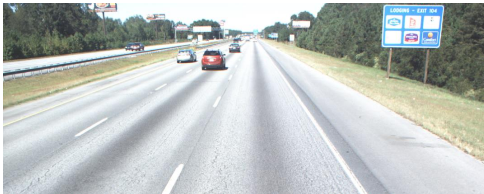
FIGURE I.14: Pavement Conditions of Test Site #3
