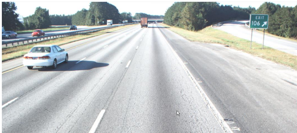
FIGURE I.22: Pavement Conditions of Test Site #10
