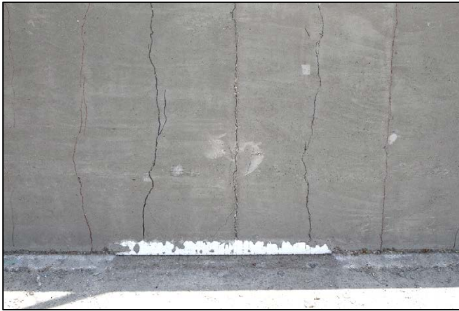
Figure 5.12. Field Side-Center of Barrier after Test No. 468957-B5.
