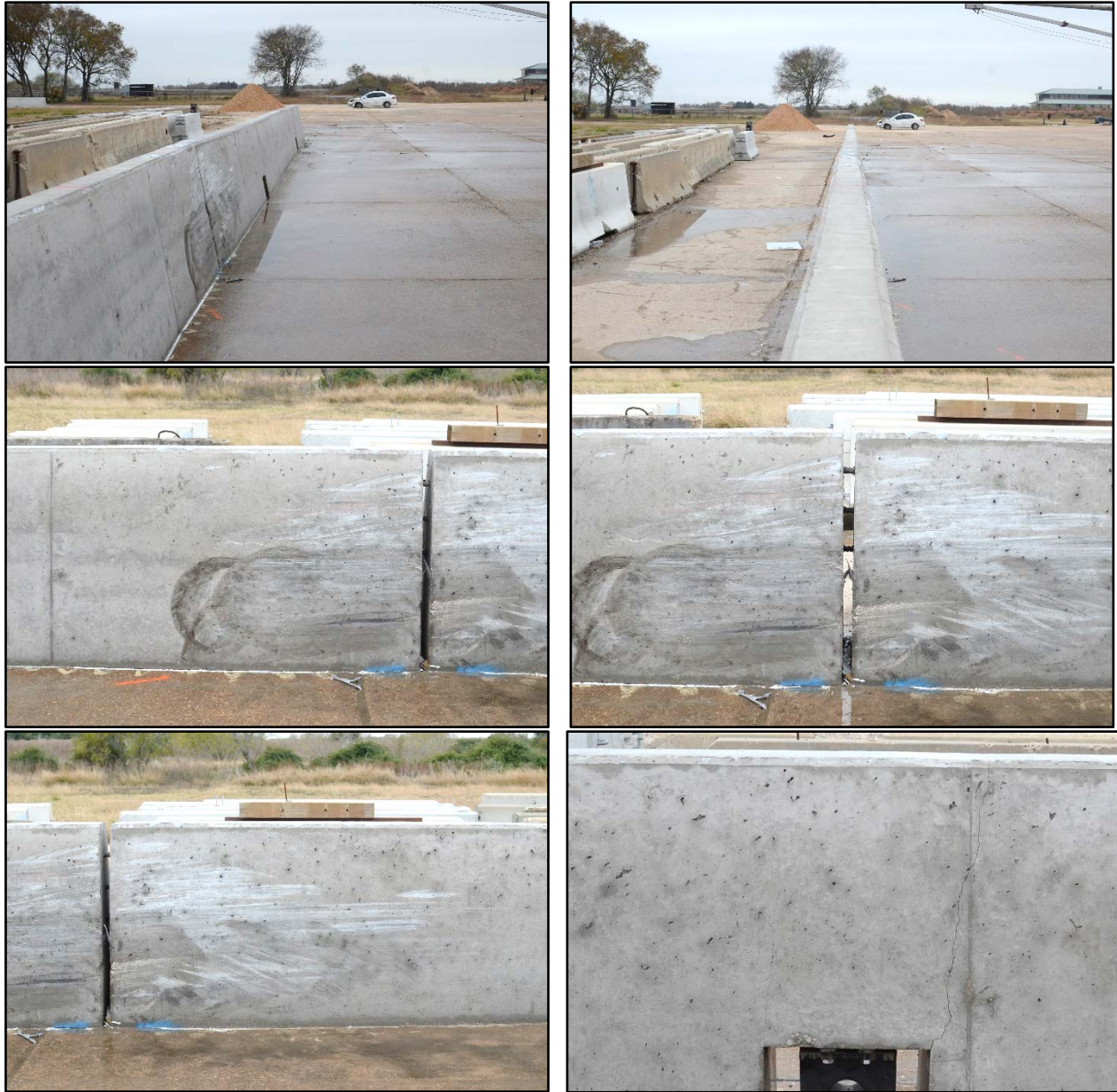
Figure 9.3. TxDOT Rubber Mounted Single Slope Barrier after Test No. 468958-3.
