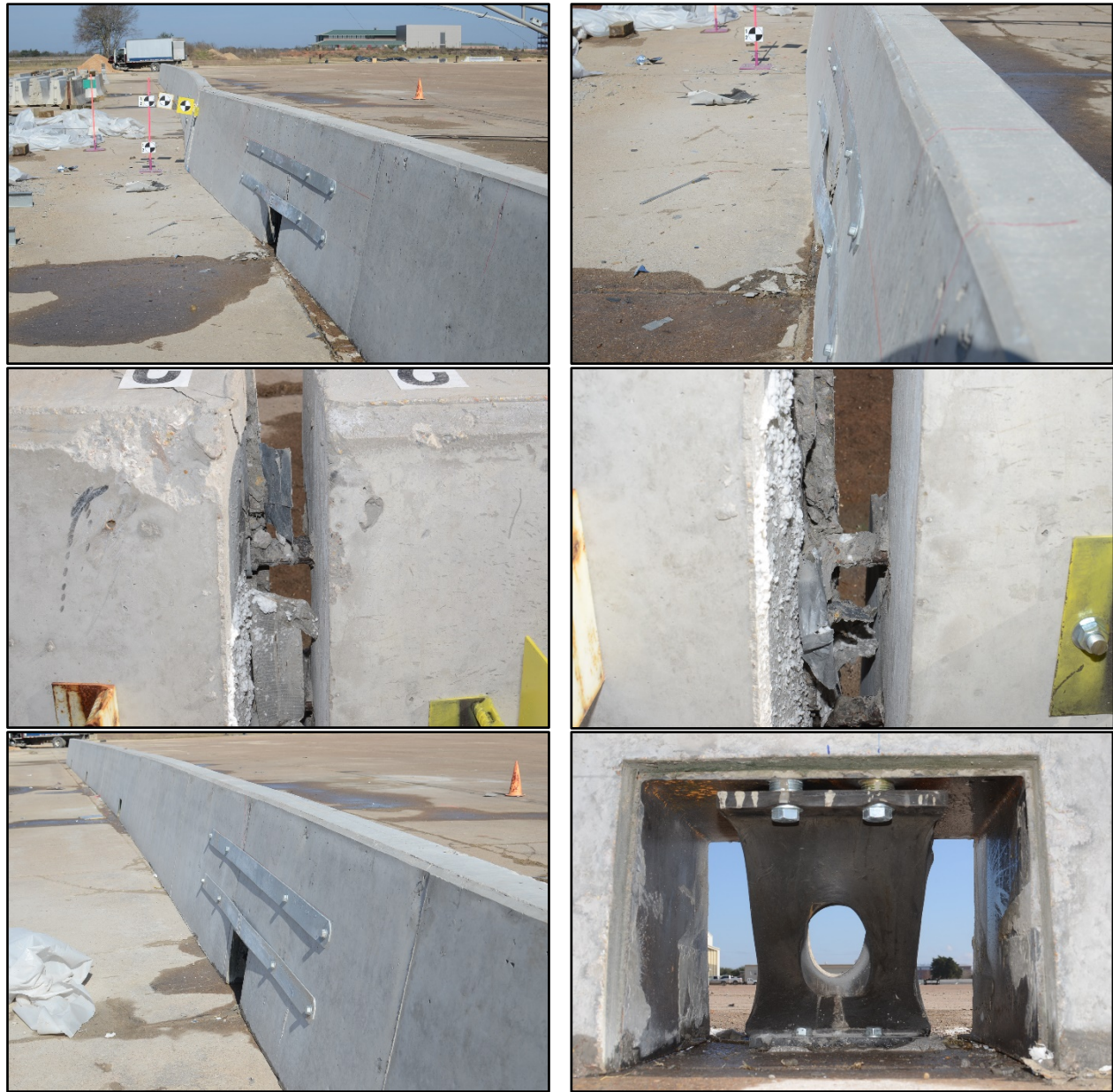
Figure 11.6. Damage to Field Side of Barrier after Test No. 468958-3.
