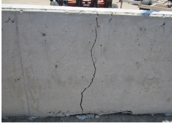
(a) CR10FGnet crack pattern
