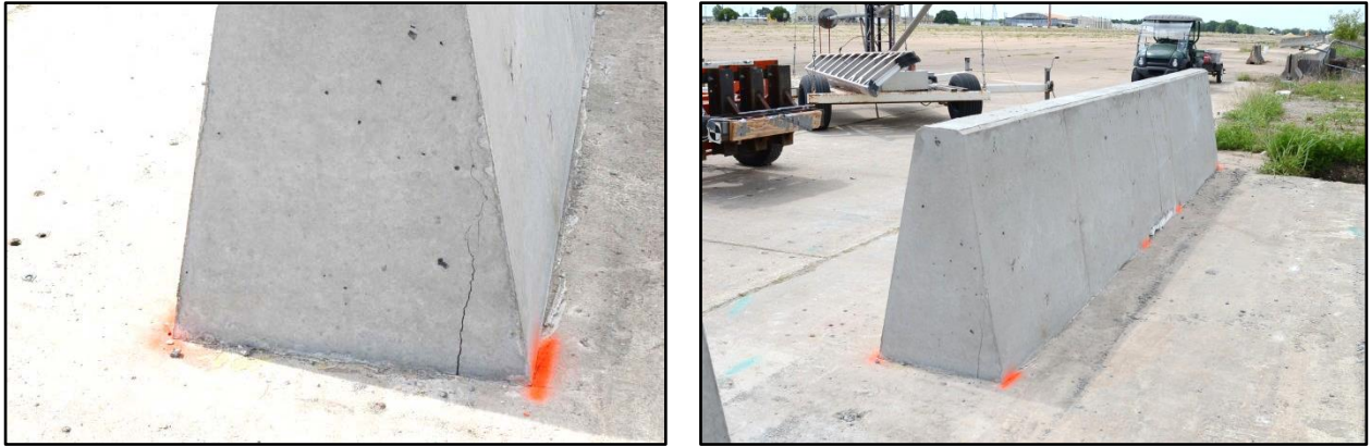
Figure 5.29. Right End and Field Side of Barrier after Test No. 468957-B8.
