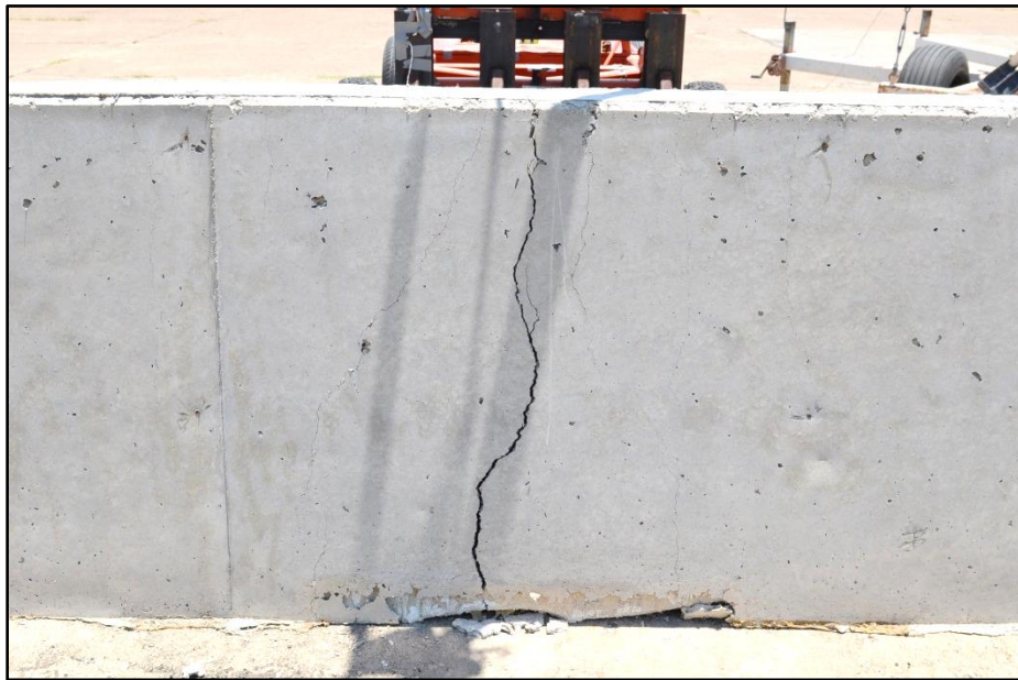
Figure 5.51. Field Side-Center of Barrier after Test No. 468957-B10.
