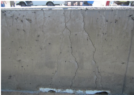
(e) PR5FCR5F crack pattern
