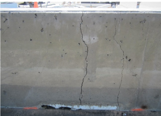
(c) Control mixture crack pattern
