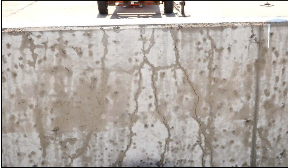
Figure 5.41. Top Field Side of Barrier after Test No. 468957-B9.
