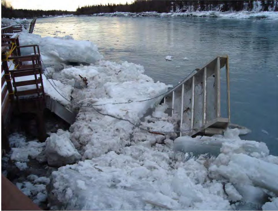
Figure 4. Damaged folding aluminum staircase at Soldotna Park. ADOT&PF photo.
