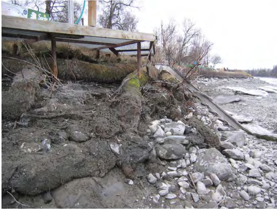
Figure 11. Ice damage to coir log installation.
