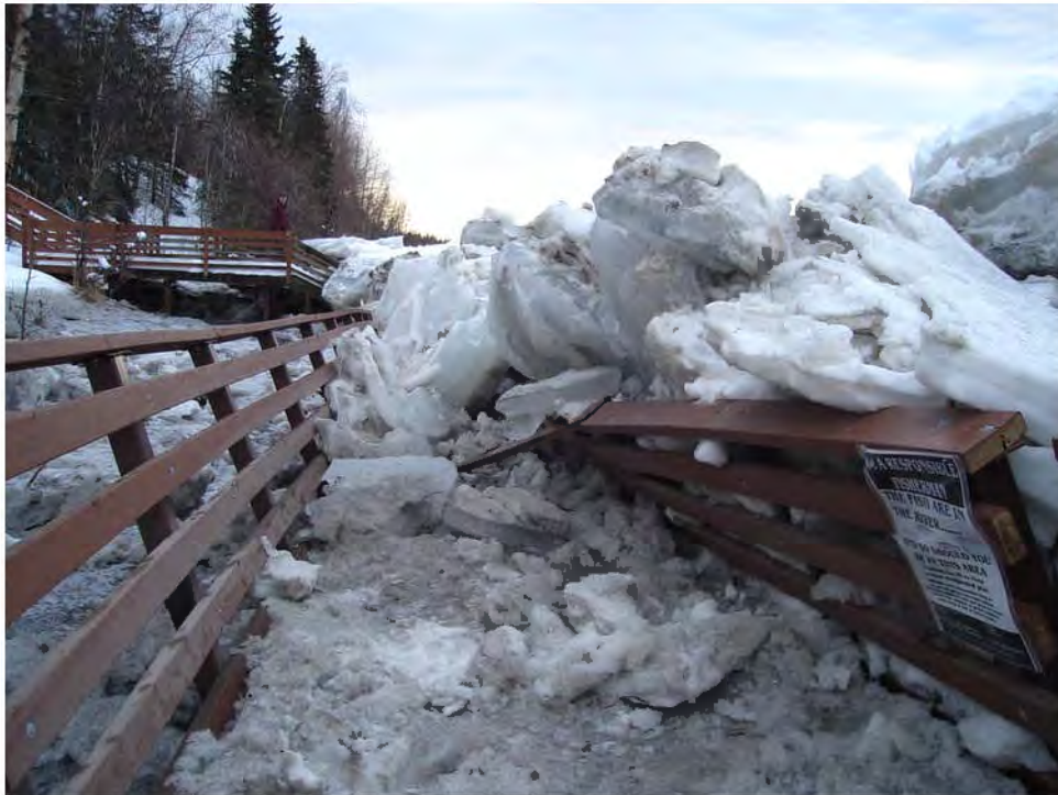
Figure 1. Elevated walk at Soldotna Park damaged by ice jam event, January 2007. ADOT&PF photo.
