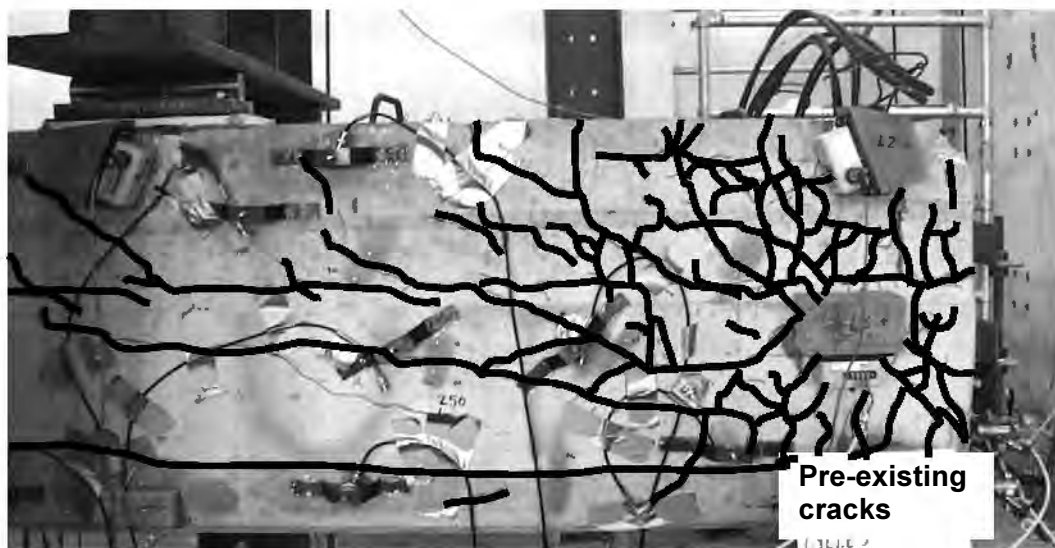
Figure 4.22 Pre-existing cracks in the west web of BG3S
