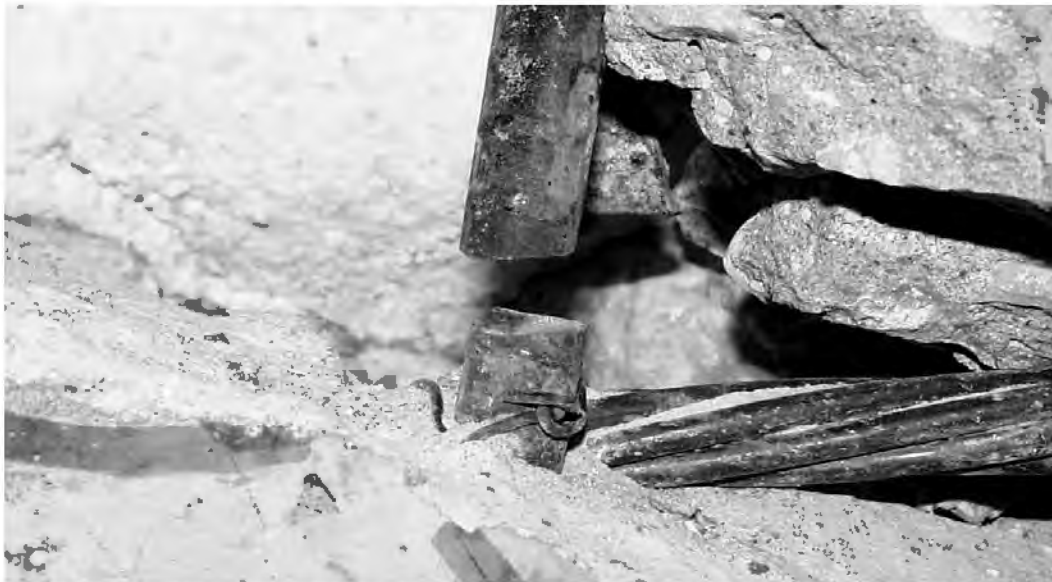
Figure 4.13 Fractured shear reinforcement (stirrup) in the east web of BG3N at failure, after removal of concrete
