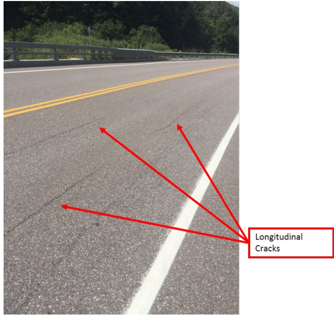
Figure 17: Longitudinal crack on northbound lane (August 15 ,2017)
