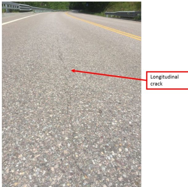
Figure 8: Longitudinal crack on southbound lane (June 2, 2016)
