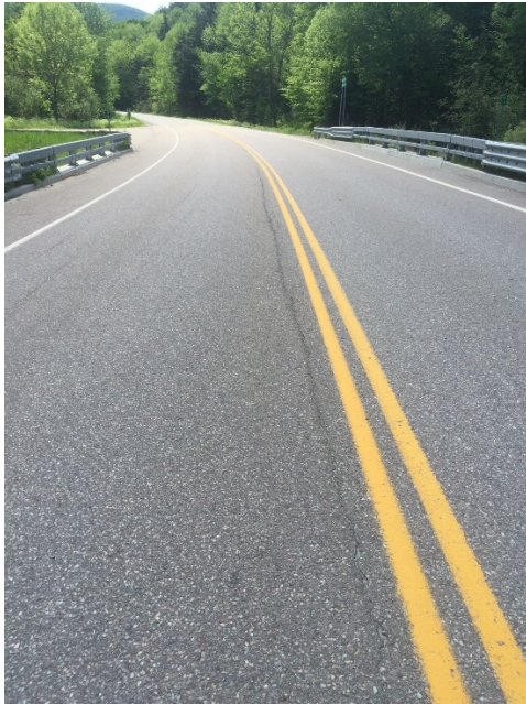
Figure 7: Centerline crack throughout bridge (June 2, 2016)
