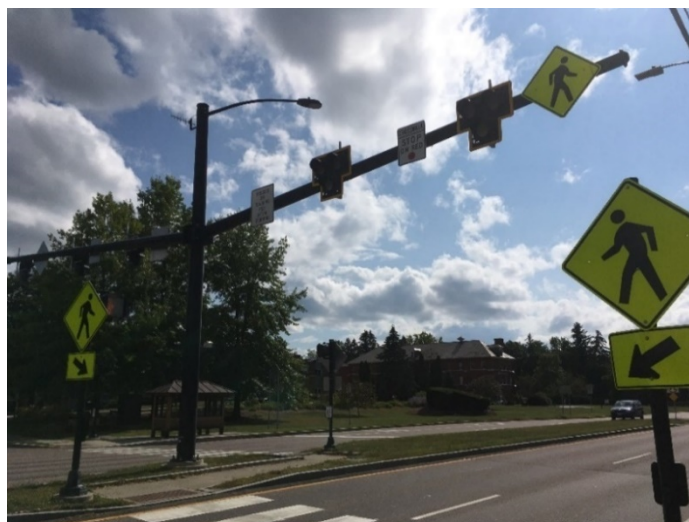
Figure 8: HAWK Crosswalk System on the westbound lane of VT Route 15 across from the Fanny Allen Hospital
