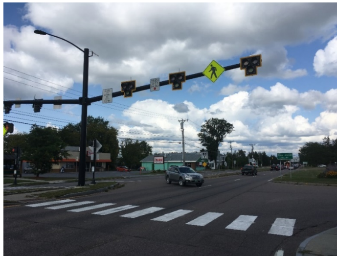
Figure 7: HAWK Crosswalk System on the eastbound lane of VT Route 15 across from the Fanny Allen Hospital
