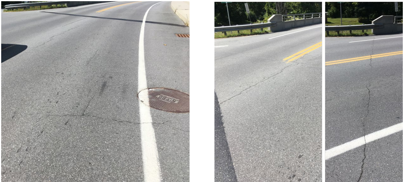
Figure 8: Cracking at eastern approach of Bridge 9
