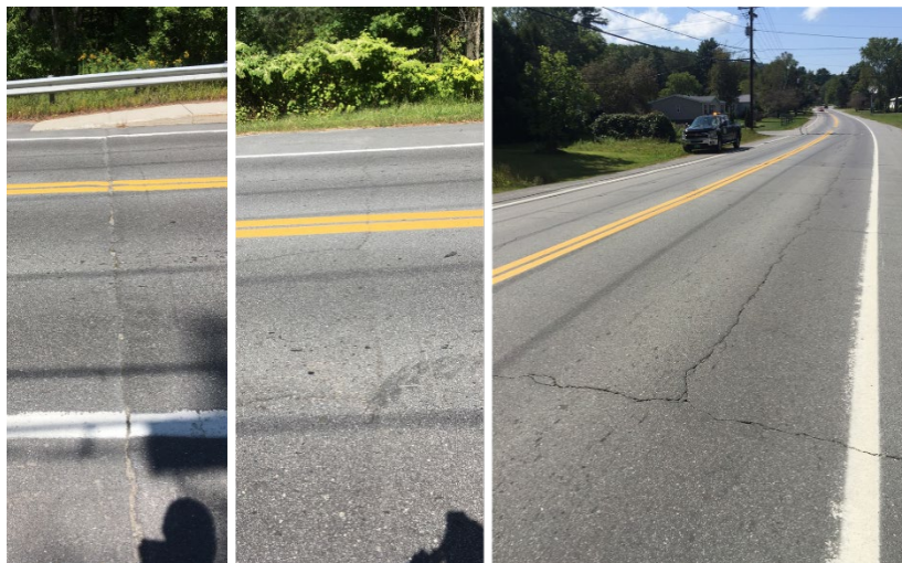
Figure 6: Cracking at western approach of Bridge 8
