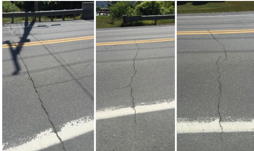
Figure 5: Cracking at eastern approach of Bridge 8
