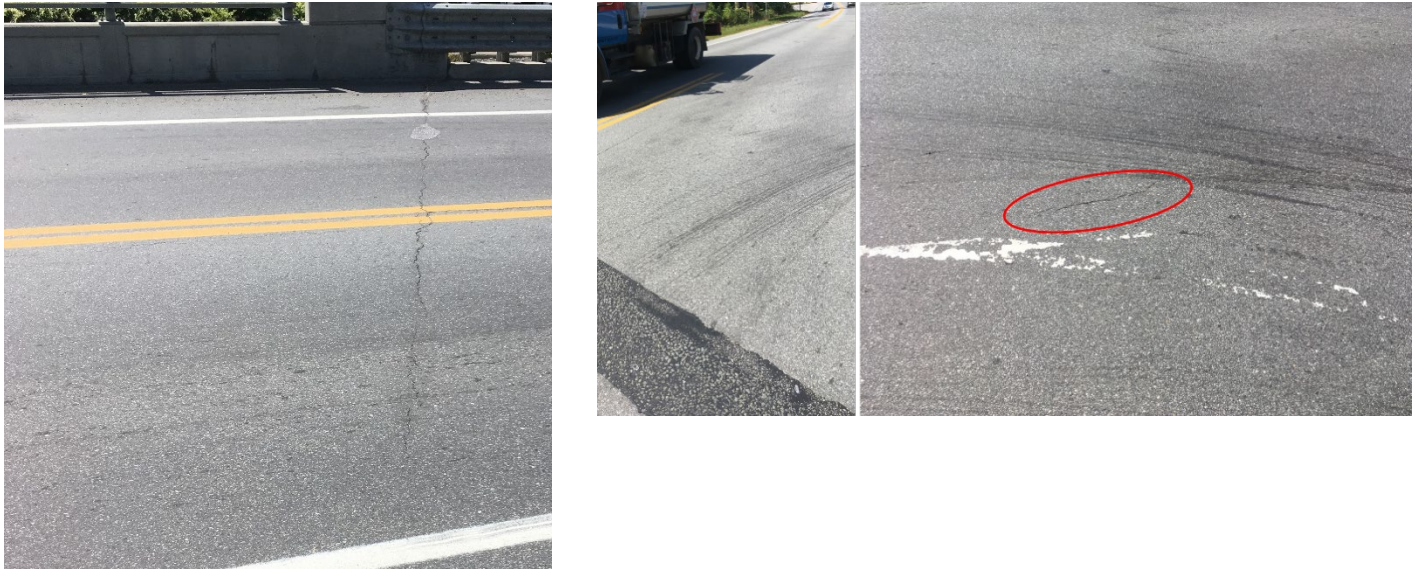
Figure 9: Cracking at the western approach of Bridge 9
