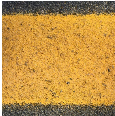
Surface Polyurea Utah, 15 months, 13-0+00
