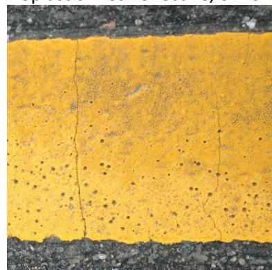
Recess Thermoplastic Wet Reflective, 8 months, 23-0+00
