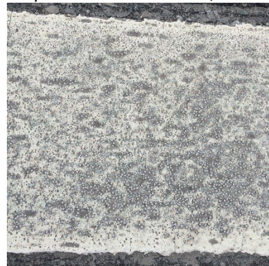
Recess Thermoplastic Wet Reflective, 8 months, 23-0+00
