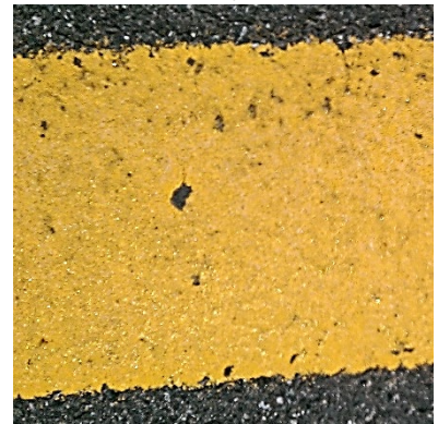
Surface Polyurea Utah, 36 months, 13-0+00
