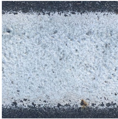
Surface Polyurea Utah, 15 months, 13-0+00
