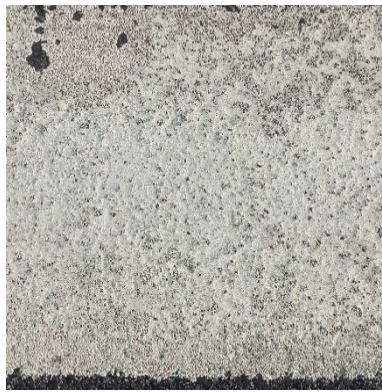
Surface Epoxy Utah, 15 months, 29-0+00
