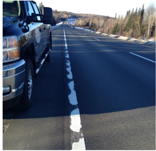
Figure 26: TS 28 Damage Overview
