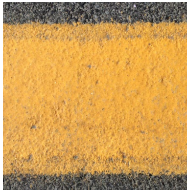
Surface Epoxy Utah, 15 months, 29-0+00
