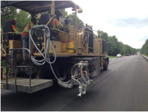
Figure 9: Polyurea application truck, featuring two chutes for application of a double drop of optics.
