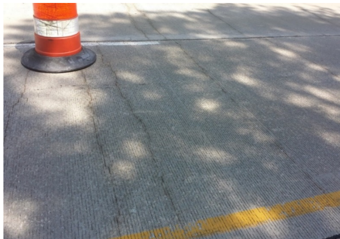
Figure 10. Five-Year-Old Patch on I-85 with Cracks Close Together. The cracks were caused by the use of concrete with a high cement content.
