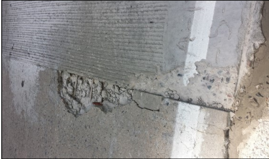
Figure 5. New Patch ( right ) Next to 40-Year-Old Pavement ( left ) on I-85. Pavement deterioration next to the patch suggests damage from concrete removal.
