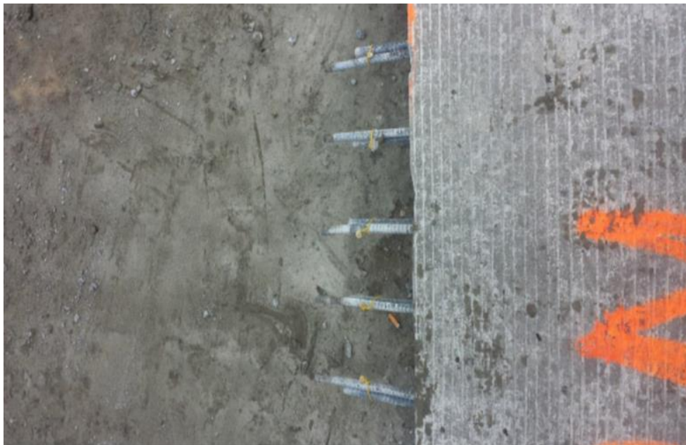
Figure 6. Single Tie Wire for Connecting Reinforcement on I-85. The 5-year-old patch that has been removed ( left ) is being replaced.
