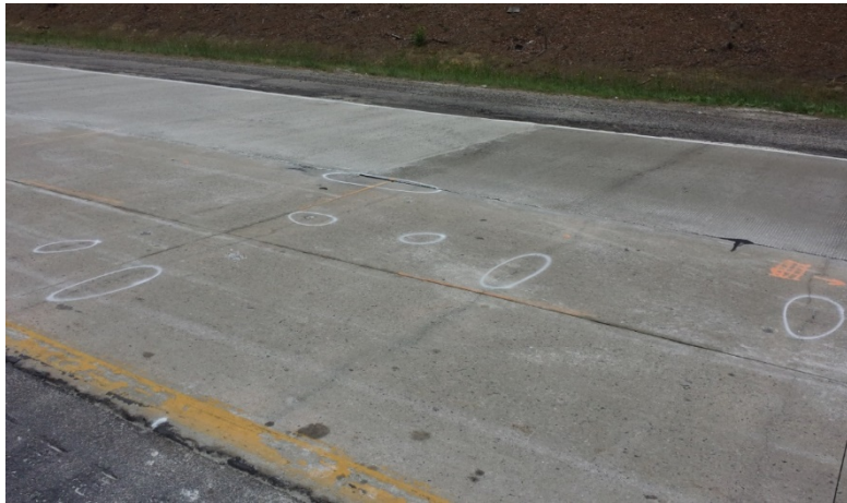
Figure 11. Section of I-85 Marked for Type IV Patching. White circles indicate spalls along cracks that justify patching the area.
