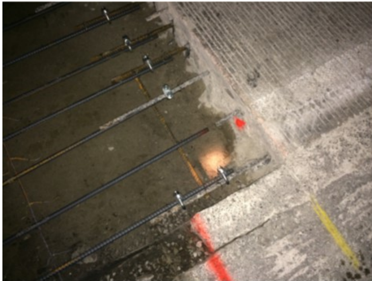
Figure 23. Exposed Reinforcement Is Absent or Too Short on SR 288
