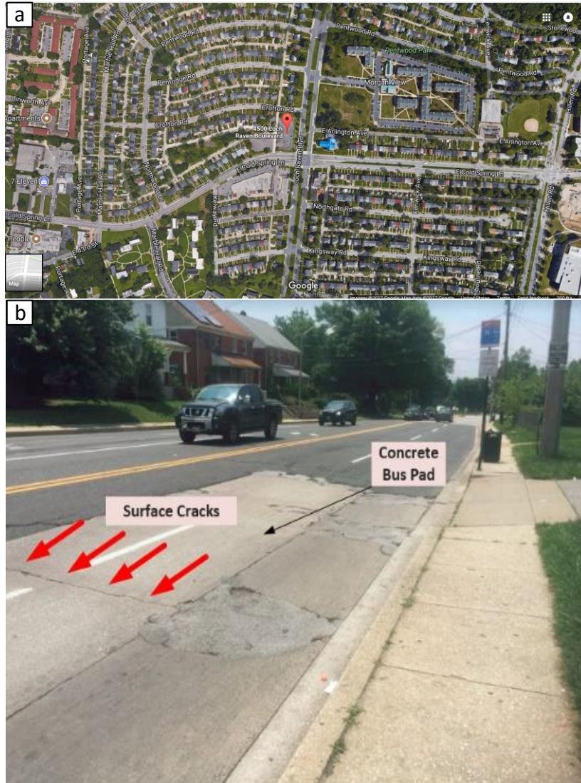
Figure 1. Field location and problem observation, (a) location of taking the field samples, (b) surface cracks were observed on concrete bus pad designed for Baltimore City
