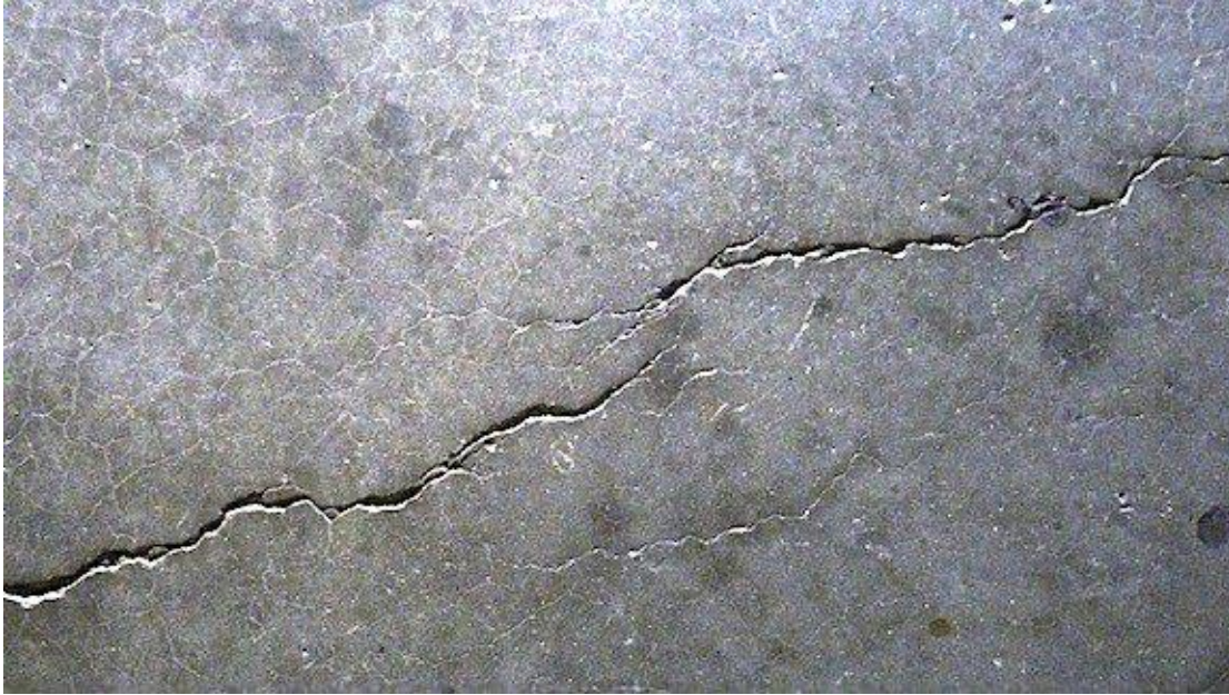
Figure 3. Concrete Shrinkage Cracking [21]
