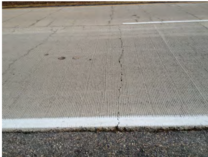
Figure 19. Cracks on 4-in Bonded Overlay on I-85
