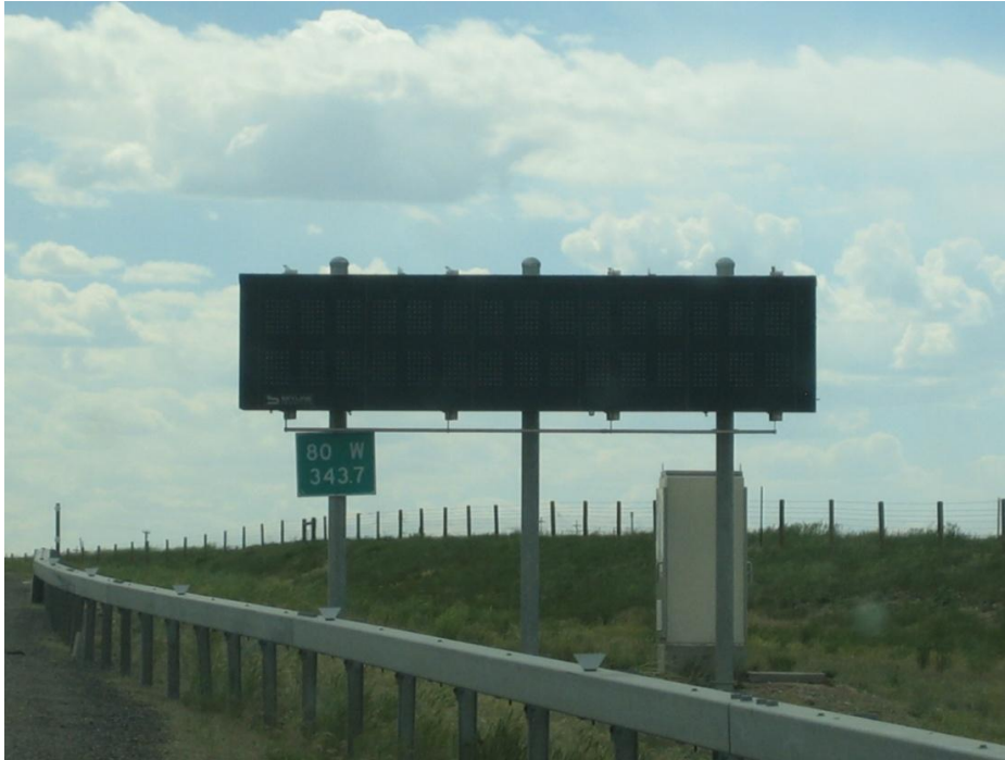
Figure 3.5 Two Line, Side Mounted DMS on I-80
